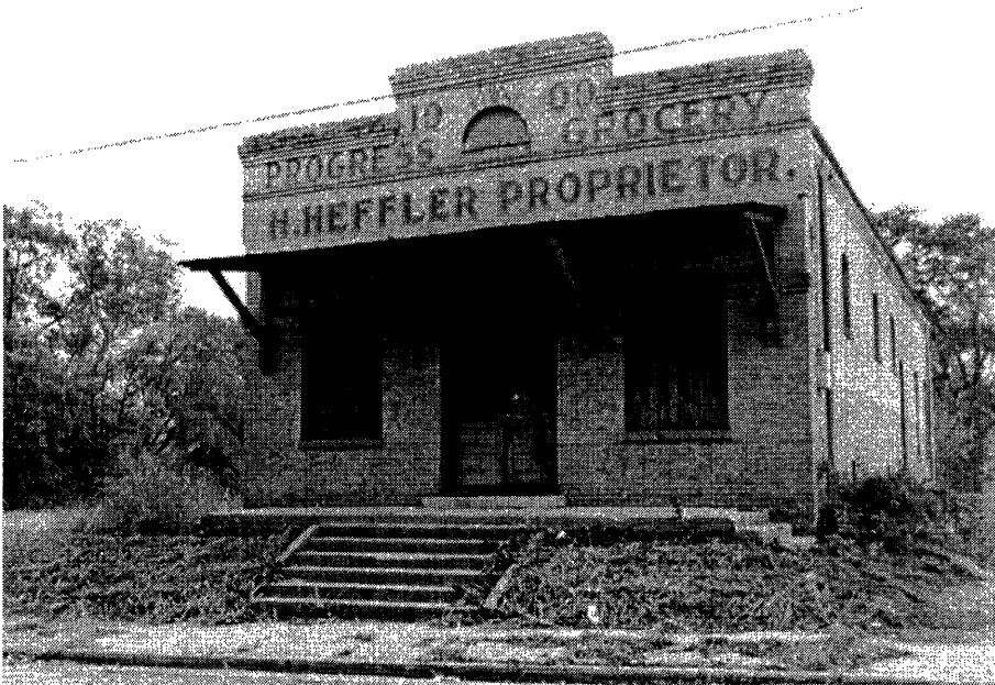
Figure 129: 1005 North Bois D'Arc Avenue, One-Part Commercial Block. Photo by Diane E. Williams
