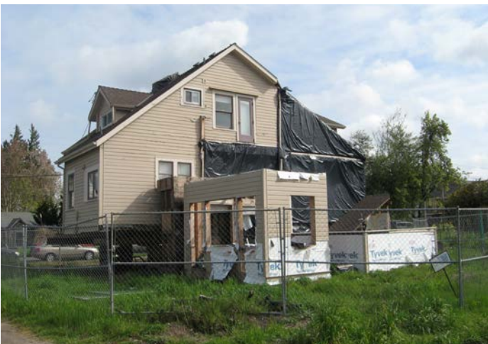
The south elevation of the building and the portions of the building that were removed for the building's move from its original location on Monroe Avenue.
