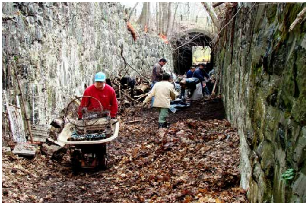
Community volunteers removed tons of debris from the tunnel along the proposed Kingston Point Rail Trail. Photo: Gregg Swanzey
