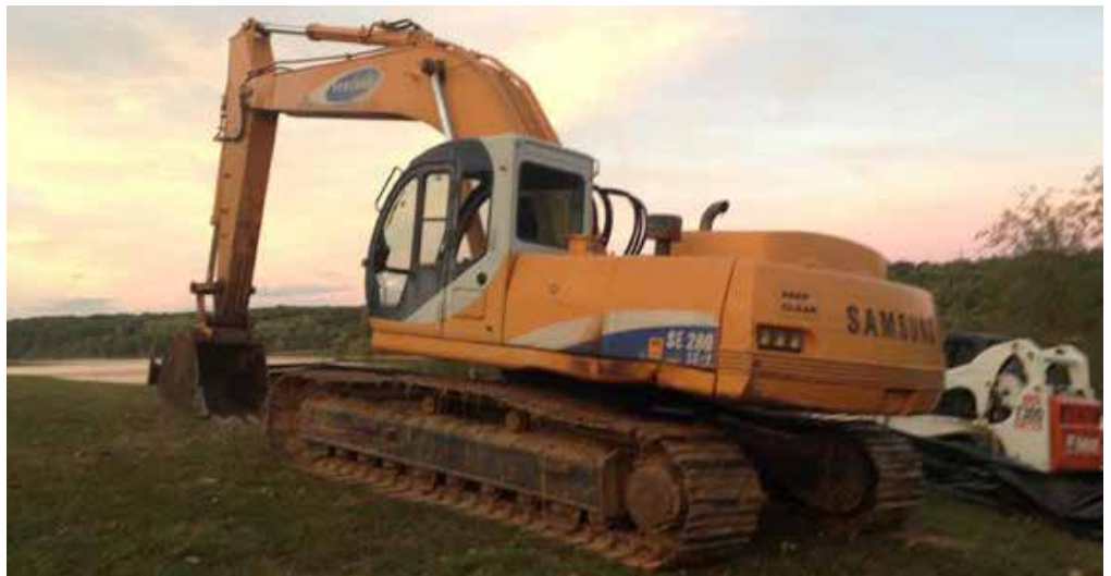
Construction begins on phase one of the Forest Lake Area Trail System at Thousand Hills State Park near Kirksville, Missouri. Photo: FLATS
