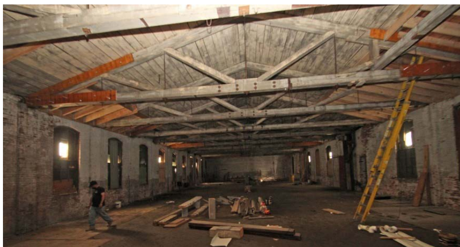
Photo 27: Fourth floor of Mill #2, view south, showing the recent reinforcement of the original roof trusses, however no other substantial changes have been made to the historic interior. Parts of the original wood floors are covered by plywood at left.
