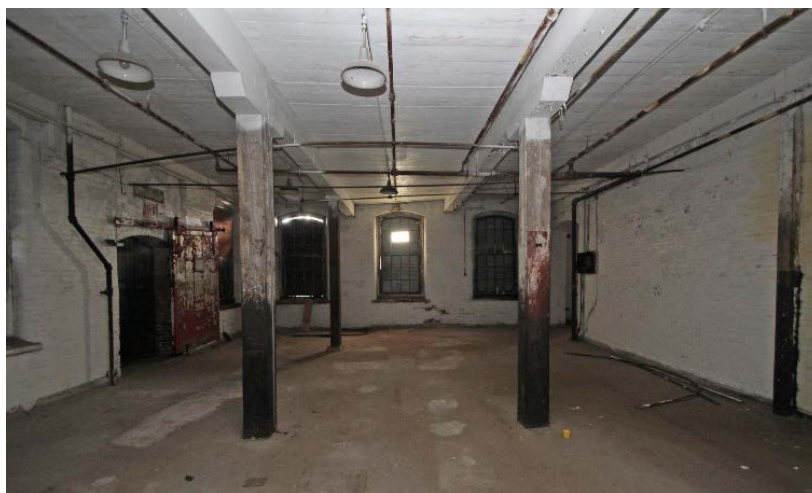
Photo 8 : Third floor of Mill #1. In this space, the floors have been covered with a gypsum concrete surface. All other materials and structural features are original.
