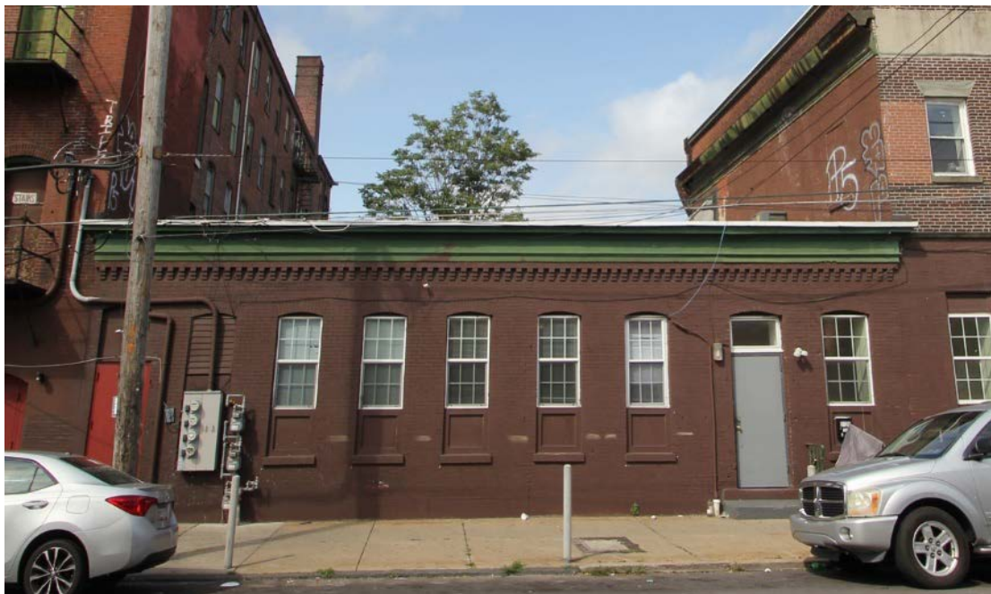
Photo 28: North elevation of the Office building, view south. The two westernmost bays (far right) were not part of the original building and were likely added shortly after 1920.
