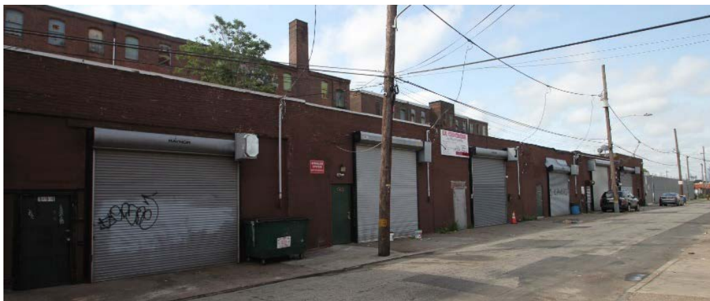
Photo 29: West elevation of the Garage building, view southeast. It appears, this elevation once contained smaller openings with windows rather than the garage doors that exist today (the doors were likely installed after 1950). As
