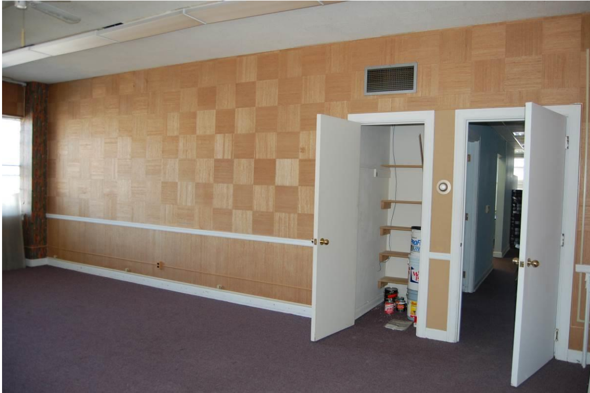
Figure 3. This area, currently used for storage (Photo 2012) illustrates an original wall finish and carpeted terrazzo floor.
