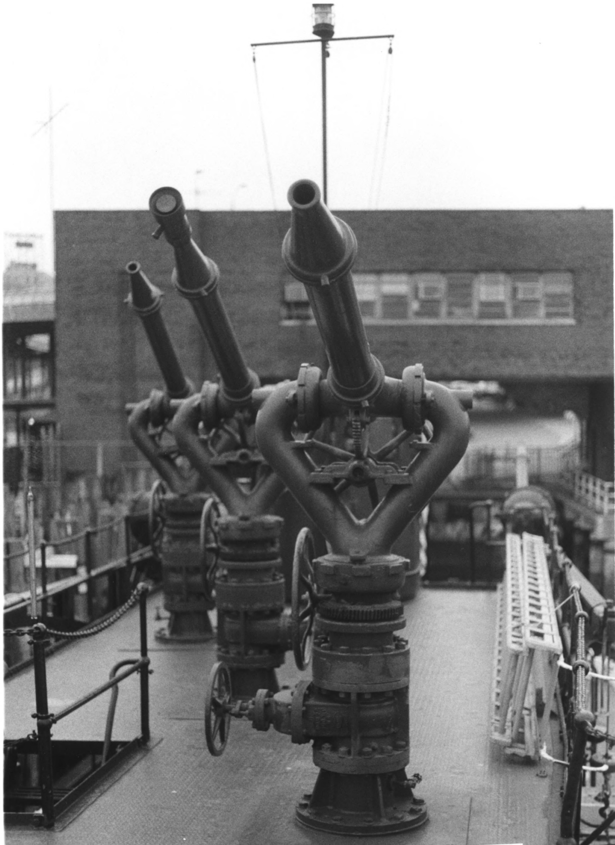
FIREBOAT FIRE FIGHTER NEW YORK, NEW YORK Owner: FIRE DEPARTMENT OF NEW YORK MONITORS ON THE PIPE DECK, LOOKING AFT. Photo #6 by JAMES P. DELGADO, 1988 Courtesy of: NATIONAL PARK SERVICE
