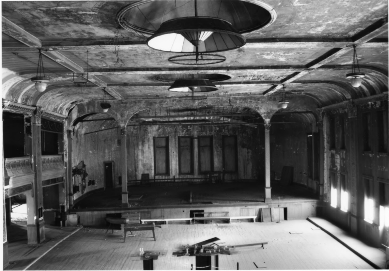
Ballroom looking East from the balcony towards the stage. Damaged in a fire on Christmas Eve 1933 and not used since. Note two original gas light chandeliers with one additional over the stage.
