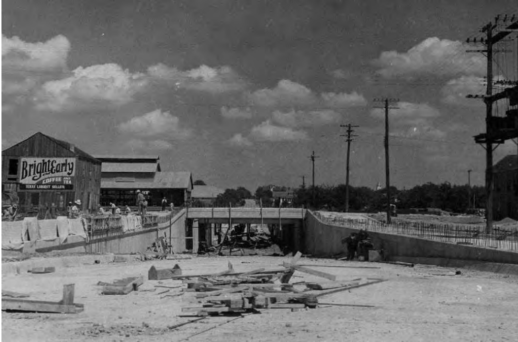
Figure 28. THD urban road and underpass construction in DeWitt County, 1936-37. (Source: Texas Department of Transportation Photo Library)
