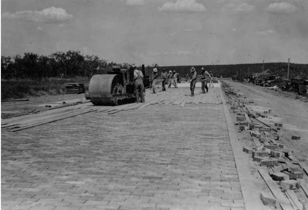
Figure 36. Installing brick pavement on US 180 in Parker and Palo Pinto Counties, 1938. At the time, the roadway was designated as Alternate US 80 and roughly followed the historic alignment of the Bankhead Highway route. (Source: Texas Department of Transportation Photo Library)
