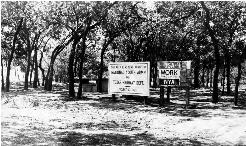
Figure 31. Joint THD/NYA roadside park construction project (Source: Texas Department of Transportation Photo Library)
