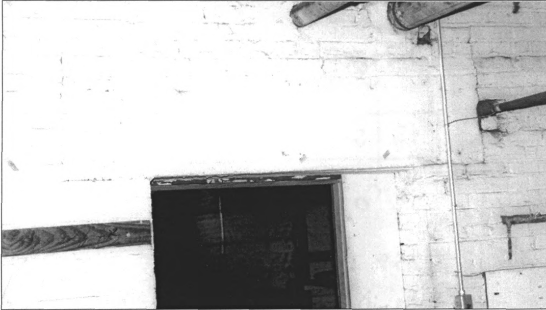
Figure 12: concrete door lintel, view northwest, basement coal room (photo by J. Jacobsen, May 26, 2006)
