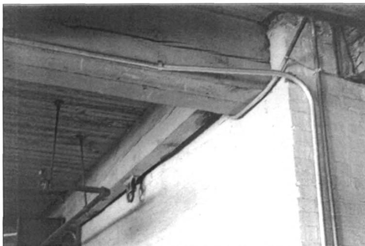
Figure 5: Primary and secondary beams are tied into the elevator enclosure, view northwest, first floor (photo by J. Jacobsen, May 26, 2006)
