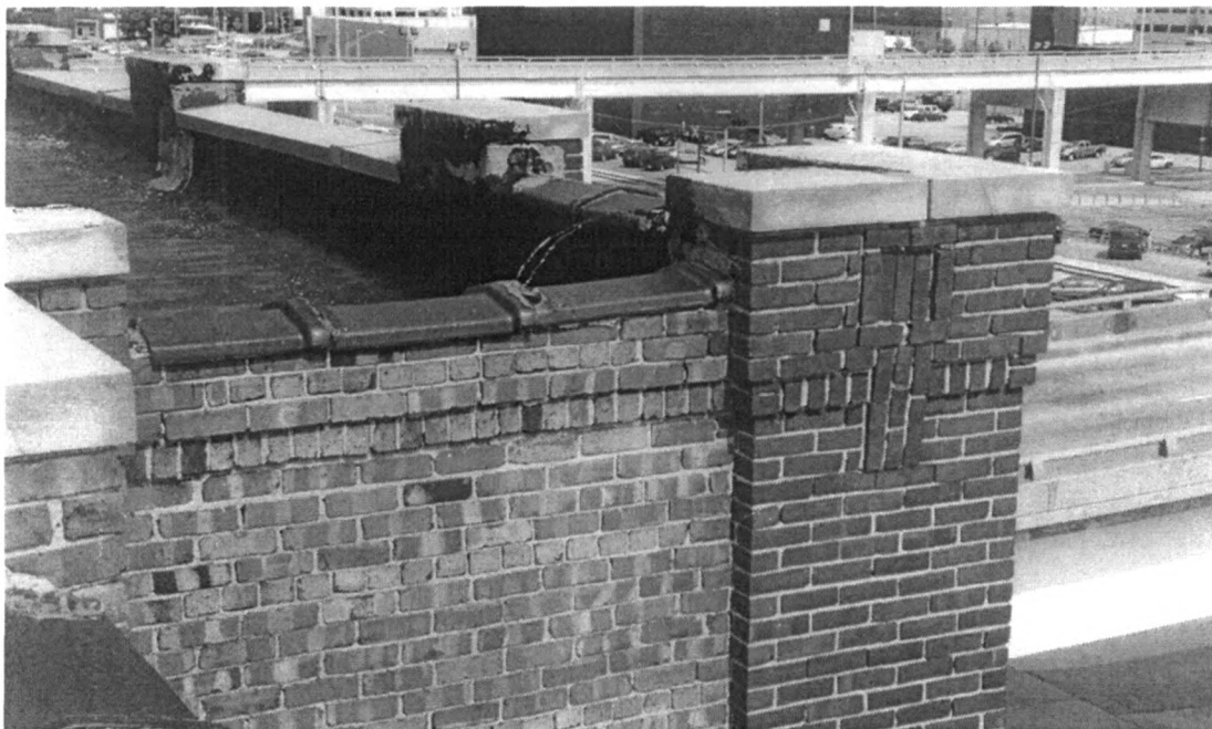
Figure 1: Cornice detail, view southeast showing parapet of south wing (photo by J. Jacobsen, May 26, 2006)
