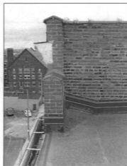
Figure 9: Parapet and cornice detail, southeast corner, view south (photo by J. Jacobsen, August 2007)
