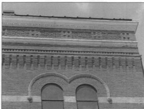
Figure 13: Supplemental photo, detail, south parapet and cornice (photo by James Jacobsen, August 9, 2007)
