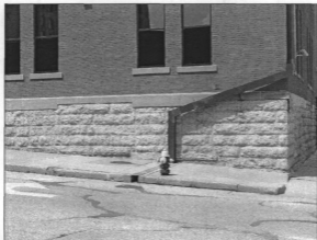
Figure 14: Supplemental photo, detail, sealed basement windows, southeast corner, view northwest (photo by James Jacobsen, August 9, 2007)
