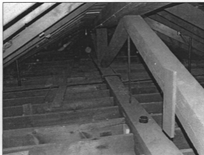
Figure 4: Truss that supported original hall ceiling and roof, view southeast (the apparent rafters are actually diagonal braces) (photo by J. Jacobsen, August 2007)
