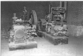
Figure 12: Ice-making equipment on first floor of brew house, view northeast (photo by J. Jacobsen, August 2006)
