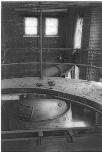
Figure 13: Brewing kettle, second floor of the brew house, view northeast from mezzanine level. (photo by J. Jacobsen, August 2006)
