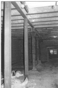
Figure 9: Steel columns in rear addition to main building, first floor, view east (photo by J. Jacobsen, August 2006)
