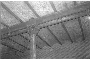
Figure 6: brick ceiling arches and steel structure, second floor, rear wing of main building, view southeast (the beams removed at the far left will allow for the construction of a central passenger elevator). (photo by J. Jacobsen, August 2006)
