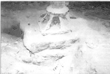
Figure 5: Exposed stone foundation support, main building, rear wing, first floor, view southwest (photo by J. Jacobsen, August 2006)
