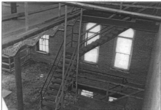
Figure 8: Multi-story void that held grain storage, view from third floor, view southeast (photo by J. Jacobsen, August 2006)
