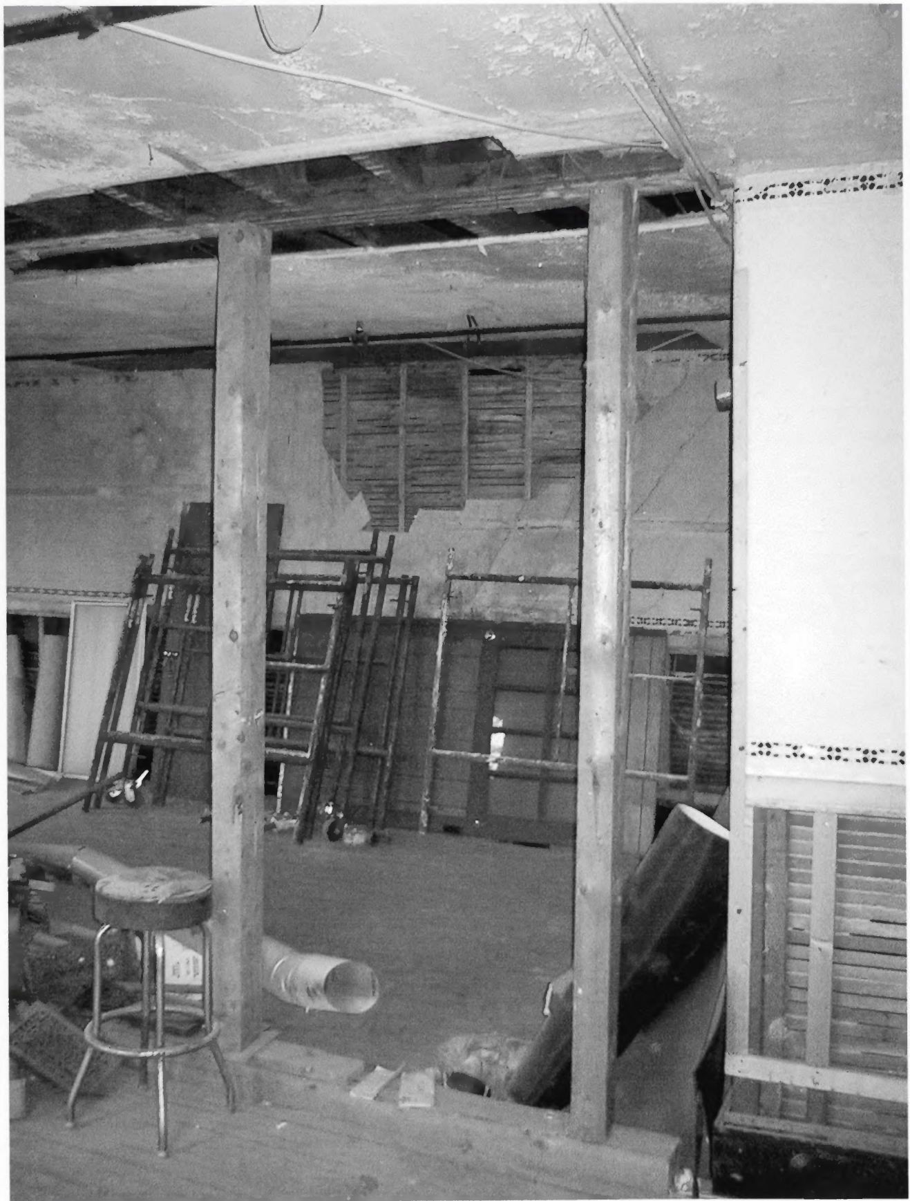
Socialist Labor Party Hall - Upstairs front room showing: temporary supports for roof timbers, damaged ceiling and wall plaster, missing wainscoting, and deteriorated paint.
