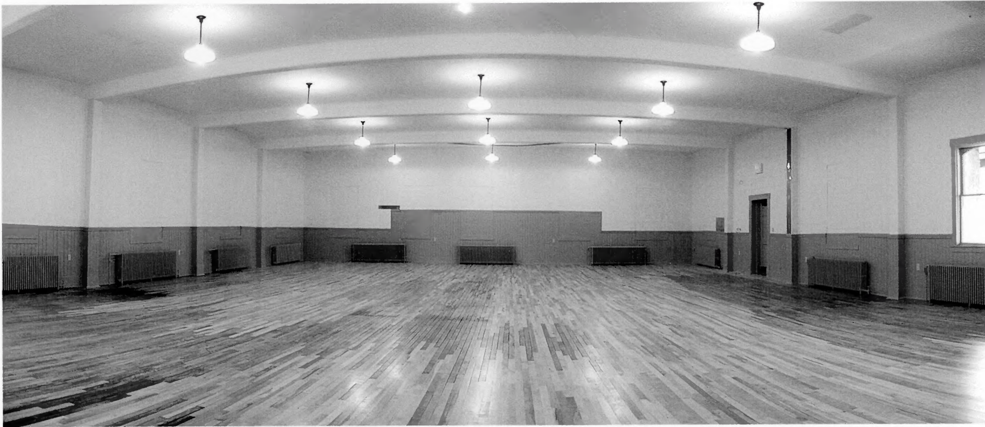
Socialist Labor Party Hall - Main meeting room after partial restoration. Work to be completed includes restoration of stage and wings at far end, replacement of bricked in window at back and sides, and repainting in original finishes of blue, red and gold and stenciling.
