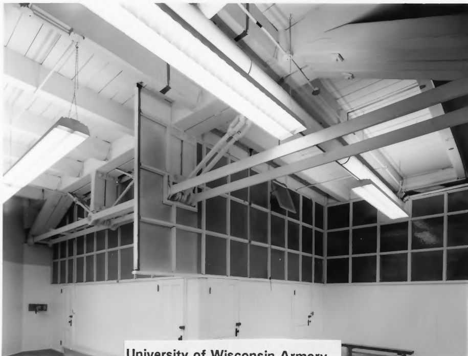
University of Wisconsin Armory and Gymnasium Madison, Dane County, WI Part of former artillery drill room Photo: Greg Gent, 1991
