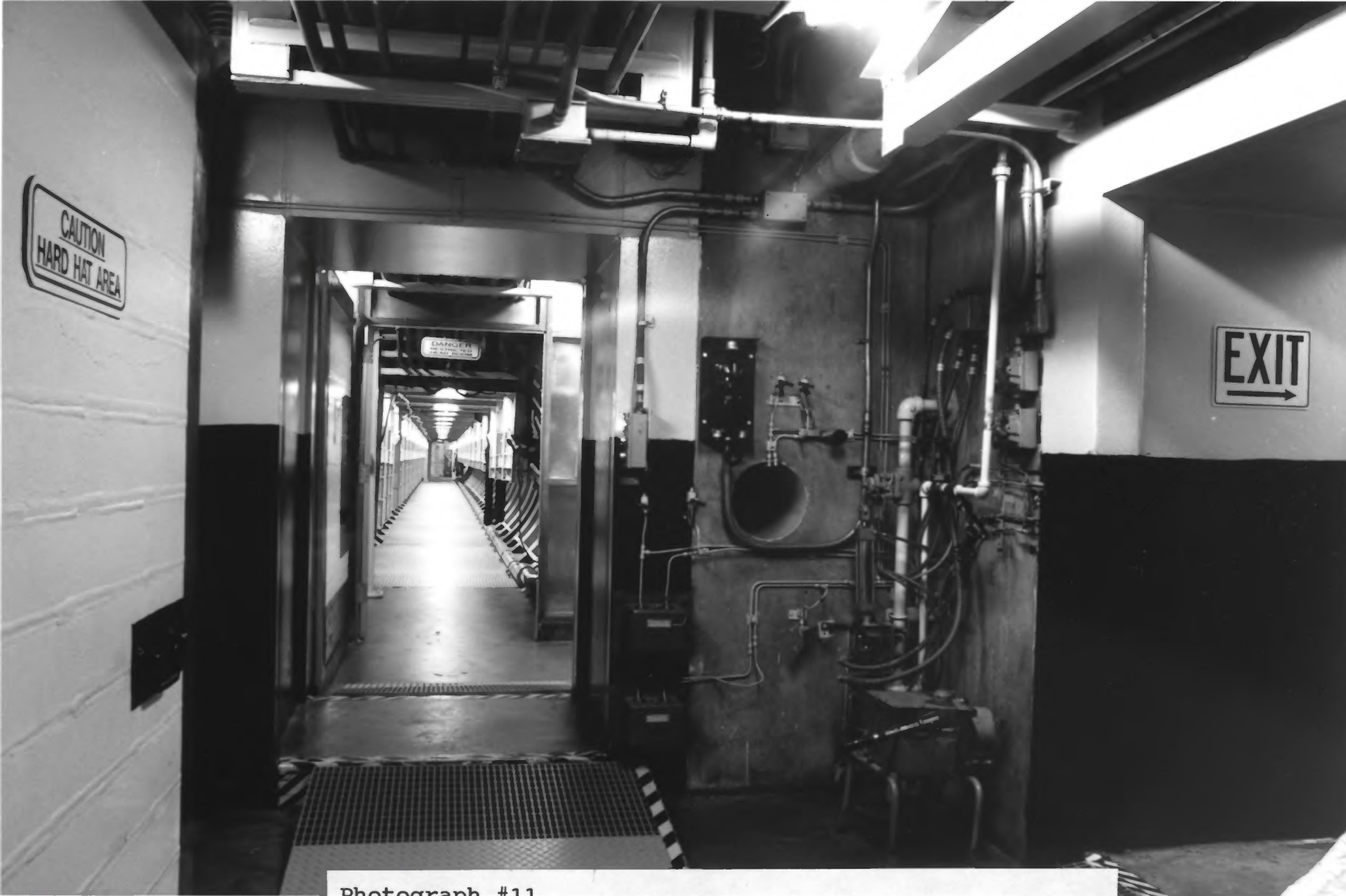
Photograph #11 Titan II ICBM Missile Site 8 (571-7) Green Valley, Pima Co., Arizona View from Blast Lock area, down 205' cableway to silo. David K. Stumpf, 1992
