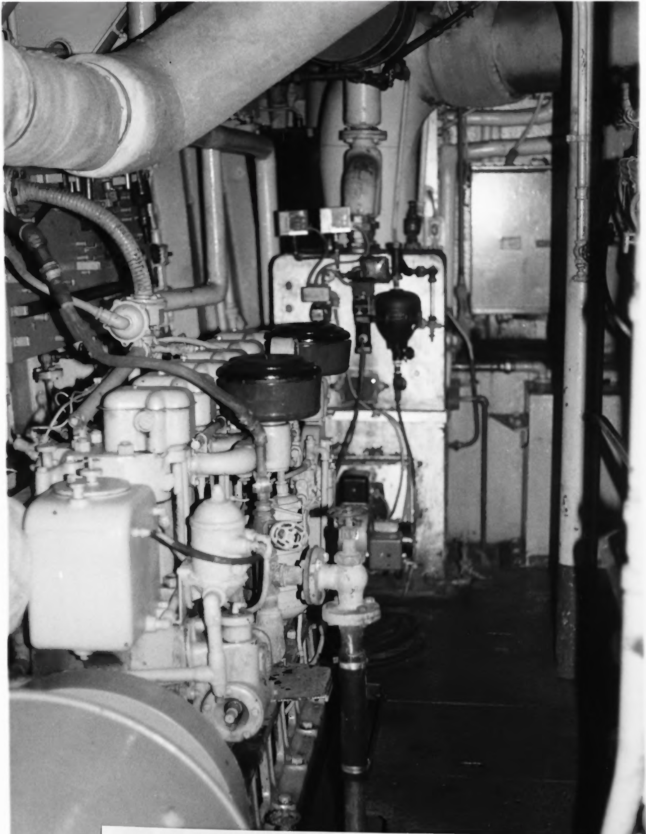
FIREBOAT CITY OF OAKLAND, EX-HOGA OAKLAND, CALIFORNIA Owner: UNITED STATES NAVY ENGINEROOM, SHOWING ORIGINAL 1940 PUMPS AND EQUIPMENT.
