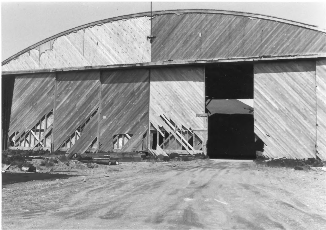
8. Deteriorated aircraft hangar at the World War II naval air station on Adak--one of only two structures still standing at the former station. This general area today is the site of several classified installations.
