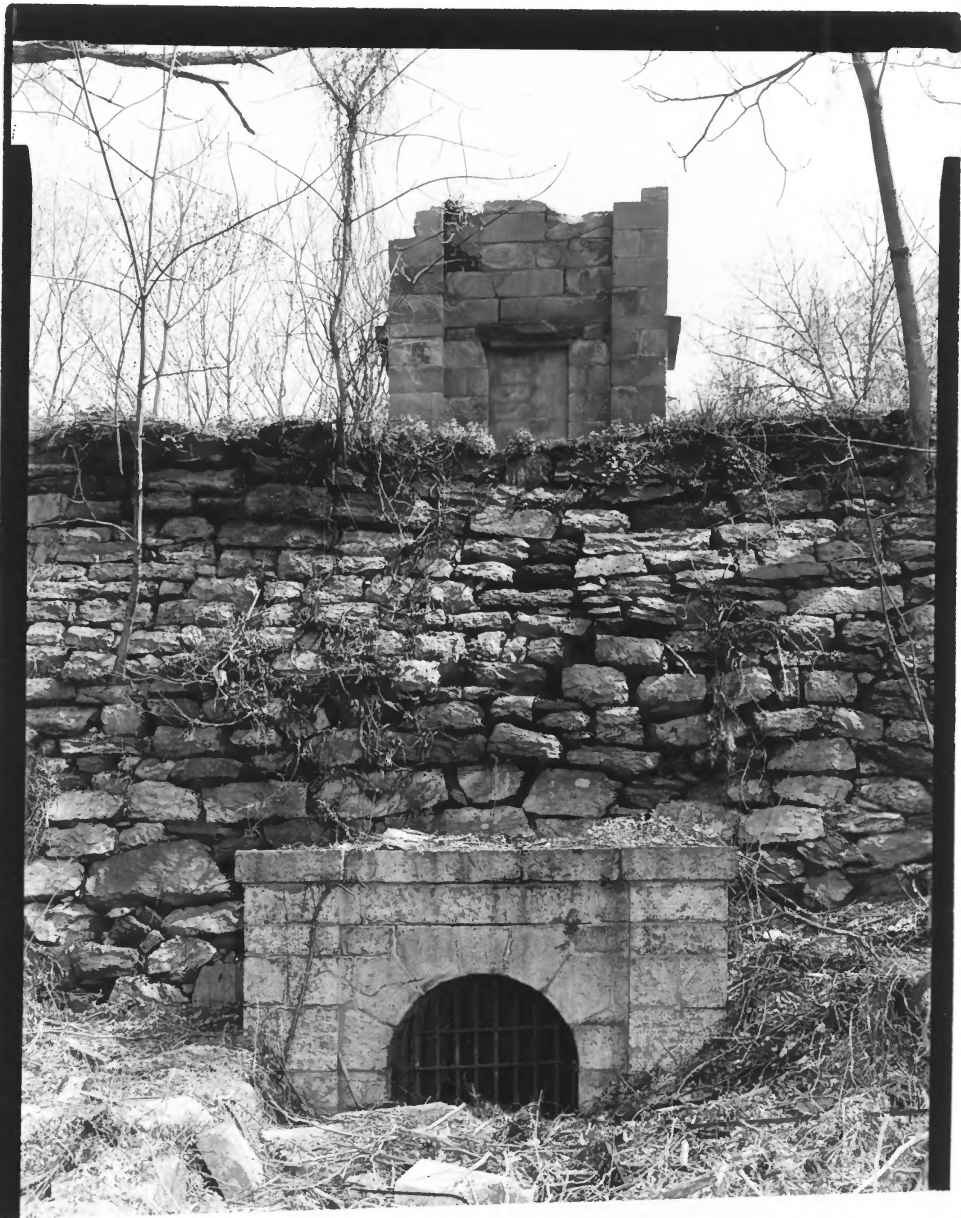
PHOTOGRAPH #9 Croton Aqueduct Ossining, New York Western elevation of the waste weir atop the Aqueduct and its discharge conduit at Snowden Avenue and Van Wyck Street in Ossining. Jack Boucher, 1978, HAER Photo No. NY-109-4.
