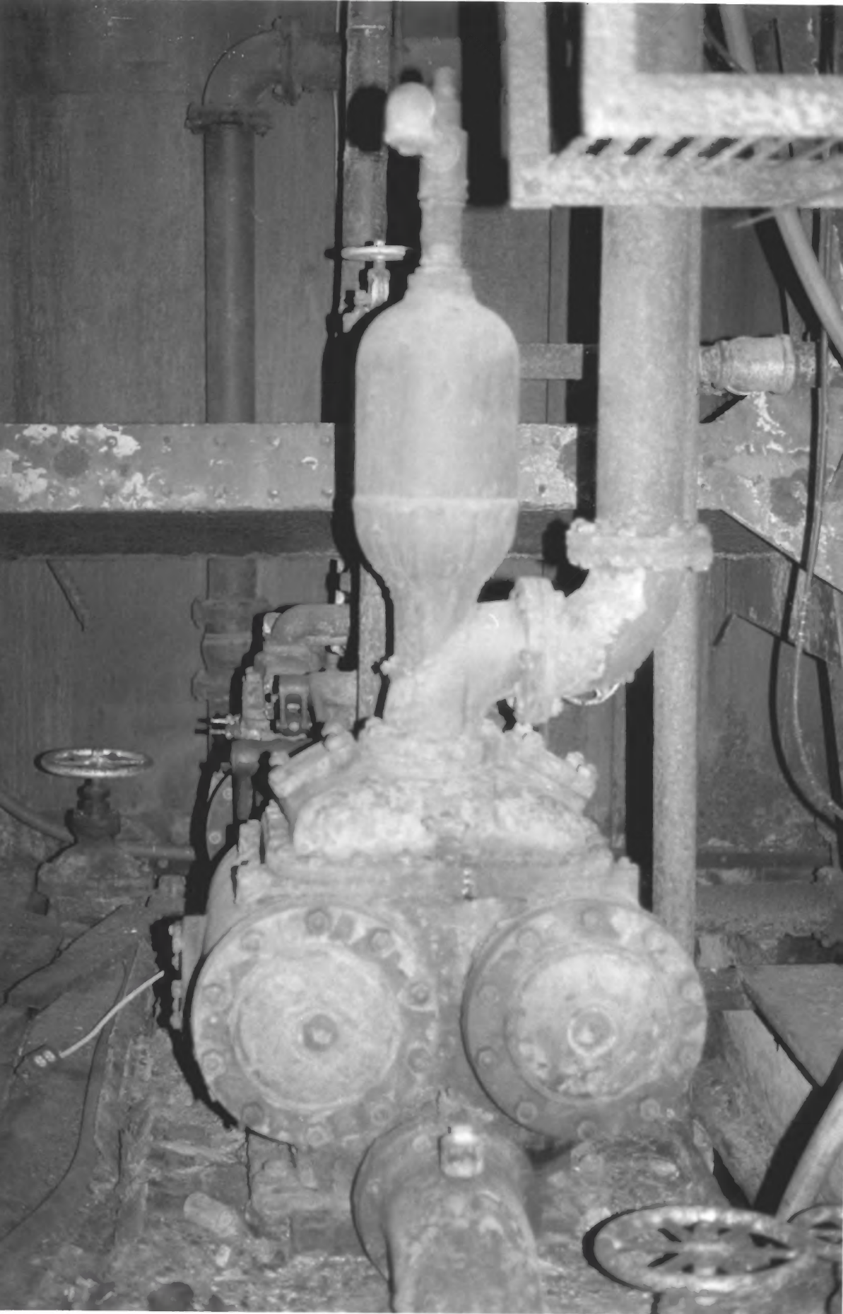
FALLS OF CLYDE , Honolulu, Hawaii National Park Service Photograph by James P. Delgado, 1988 Hawaii Maritime Center, Inc. Horizontal salt-water ballast pump in tanker pump room. Photo #10
