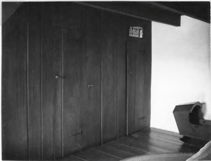
POPLAR VERTICAL SHEATHING PARTITIONS WITH OVER DOOR VENTILLATORS (TYPICAL OF S.E. PENNSYLVANIA ENGLISH TYPE HOMES OF EARLY 18TH CENTURY) CROOKS HOUSE
