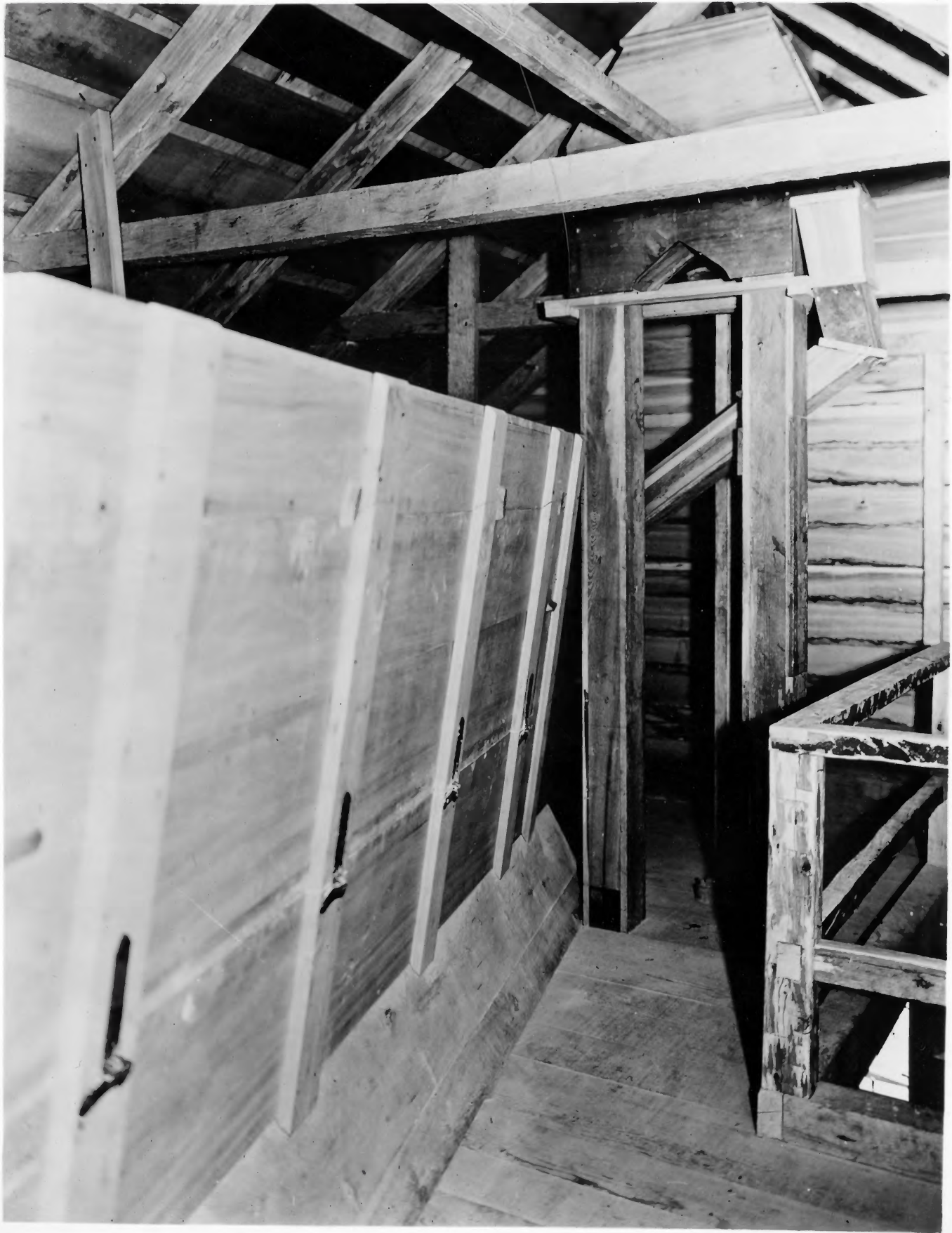
View of Interior of Mill Building, Third Floor. Bolting Chest with Door closed, Elevators and Chute.
