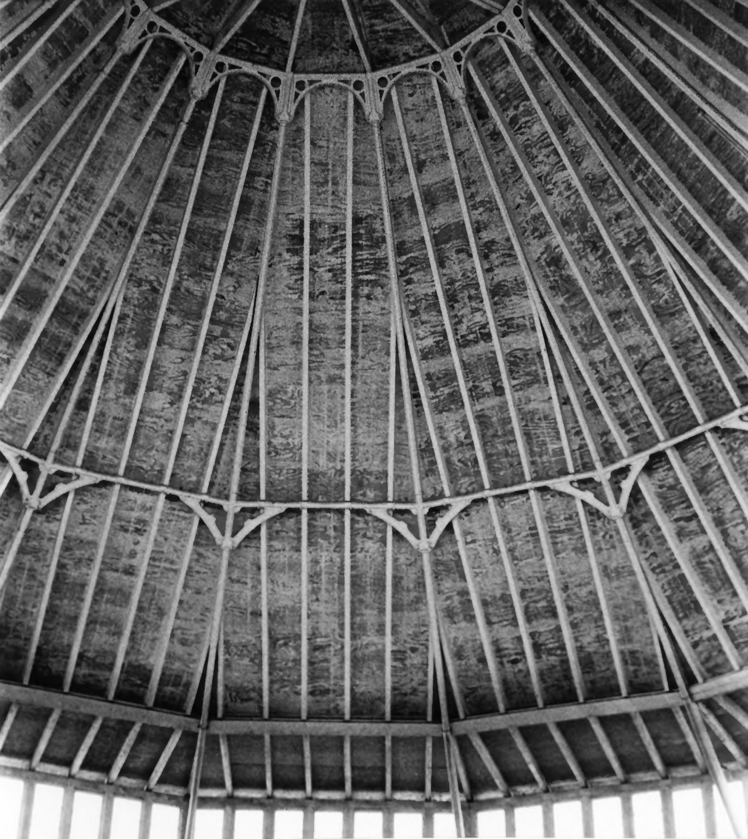
Photograph #10 B&O RAILROAD MARTINSBURG SHOPS Martinsburg, WV Interior of West Roundhouse, framework of dome, looking northeast. Michael Caplinger, IHTIA, August 2001
