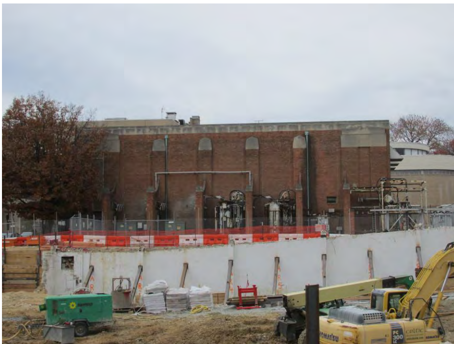
Pepco Substation No. 25
