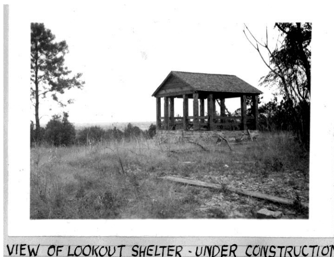
Figure 2: Shelter #5 under construction [Photo album of State Parks, 1934-1940, CCC files (photographs), State Commission of Forestry Records, SCDAH, Columbia, S.C.]
