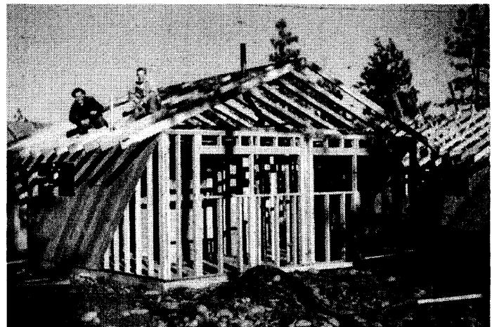
R-04: Bath house under construction Photographer: Jim Allen, 1954; Looking northeast Bath house shows position of windows and one-by-six subsiding. Barracks is under construction in background.
