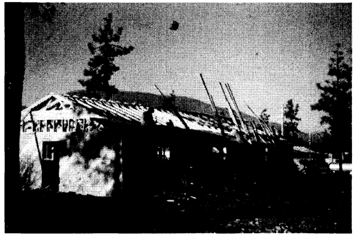
R-02: Barracks under construction Photographer: Jim Allen, 1954; Looking northwest Barracks under construction showing one-by-six subsiding that was later covered with shingles.
