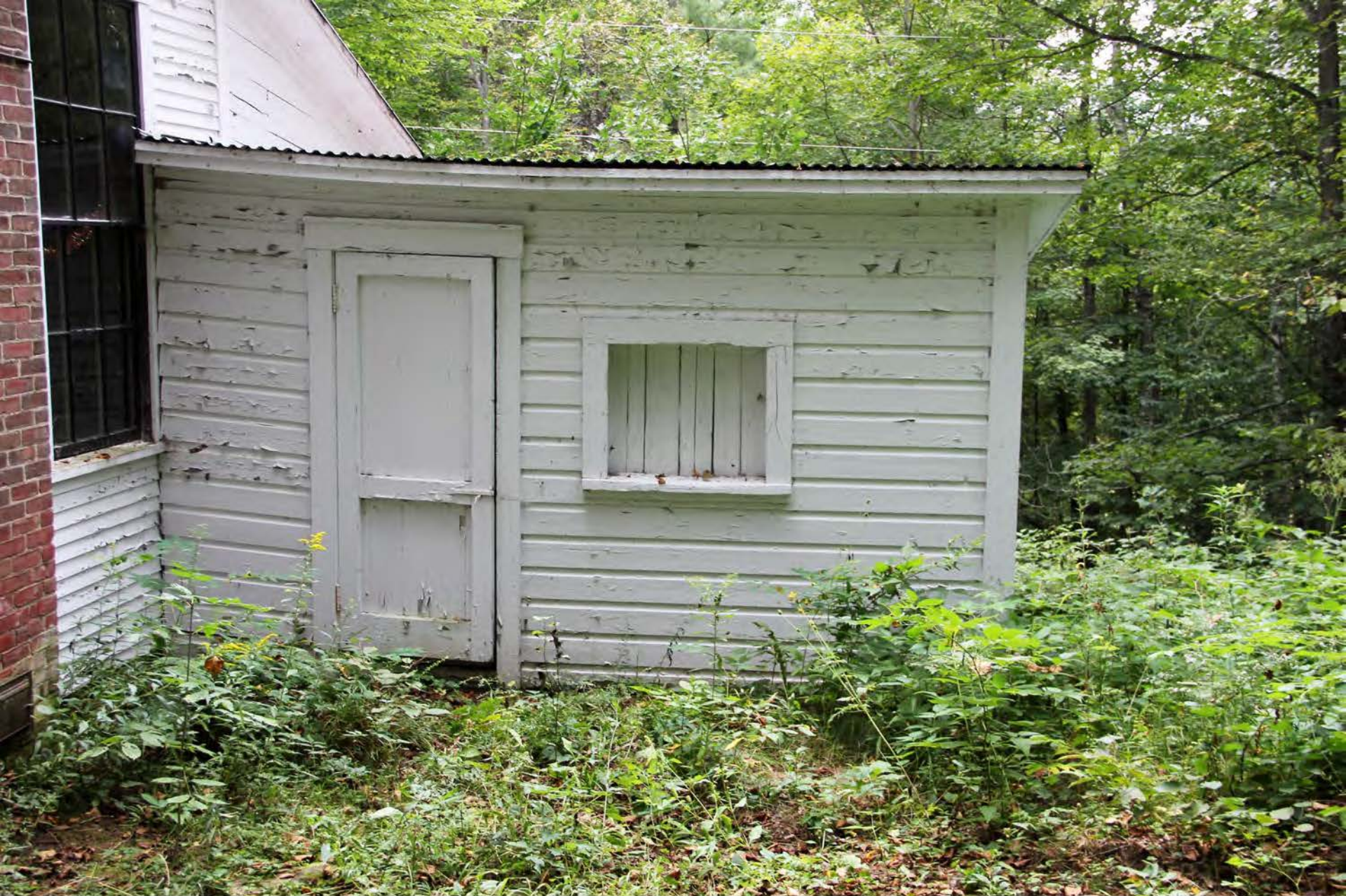
Beaver Meadow School, Norwich, Windsor Co., Vermont Photograph #11 of 16 Beaver Meadow School wood shed, east elevation, view looking west
