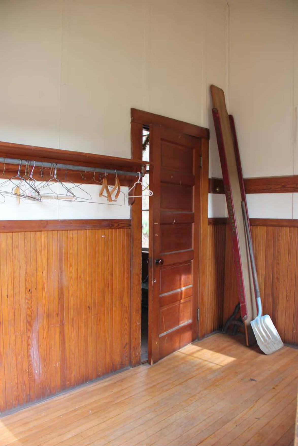
Beaver Meadow School, Norwich, Windsor Co., Vermont Photograph #12 of 16 Cloakroom, view looking northeast
