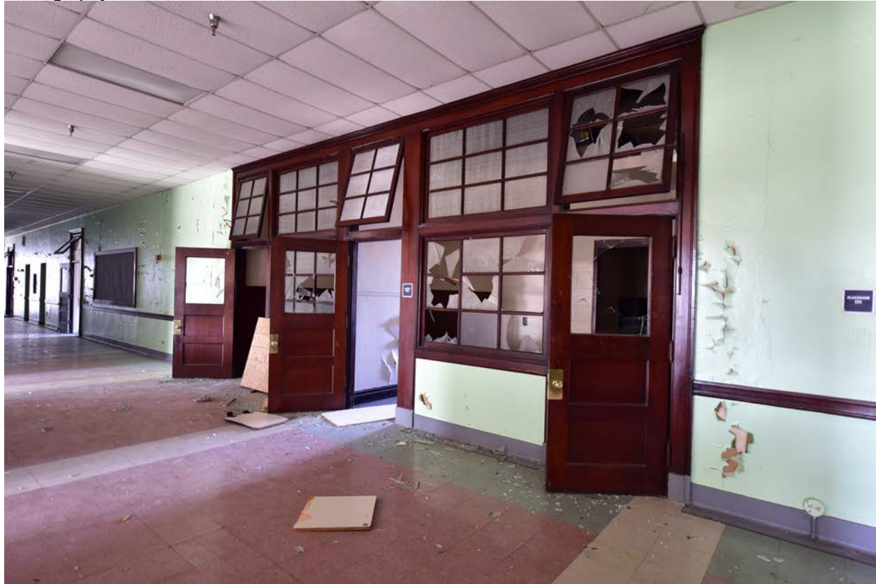
Figure 20. Photo of historic window wall on north side of second-floor corridor. Source: f-stop Photography, December 2020.
