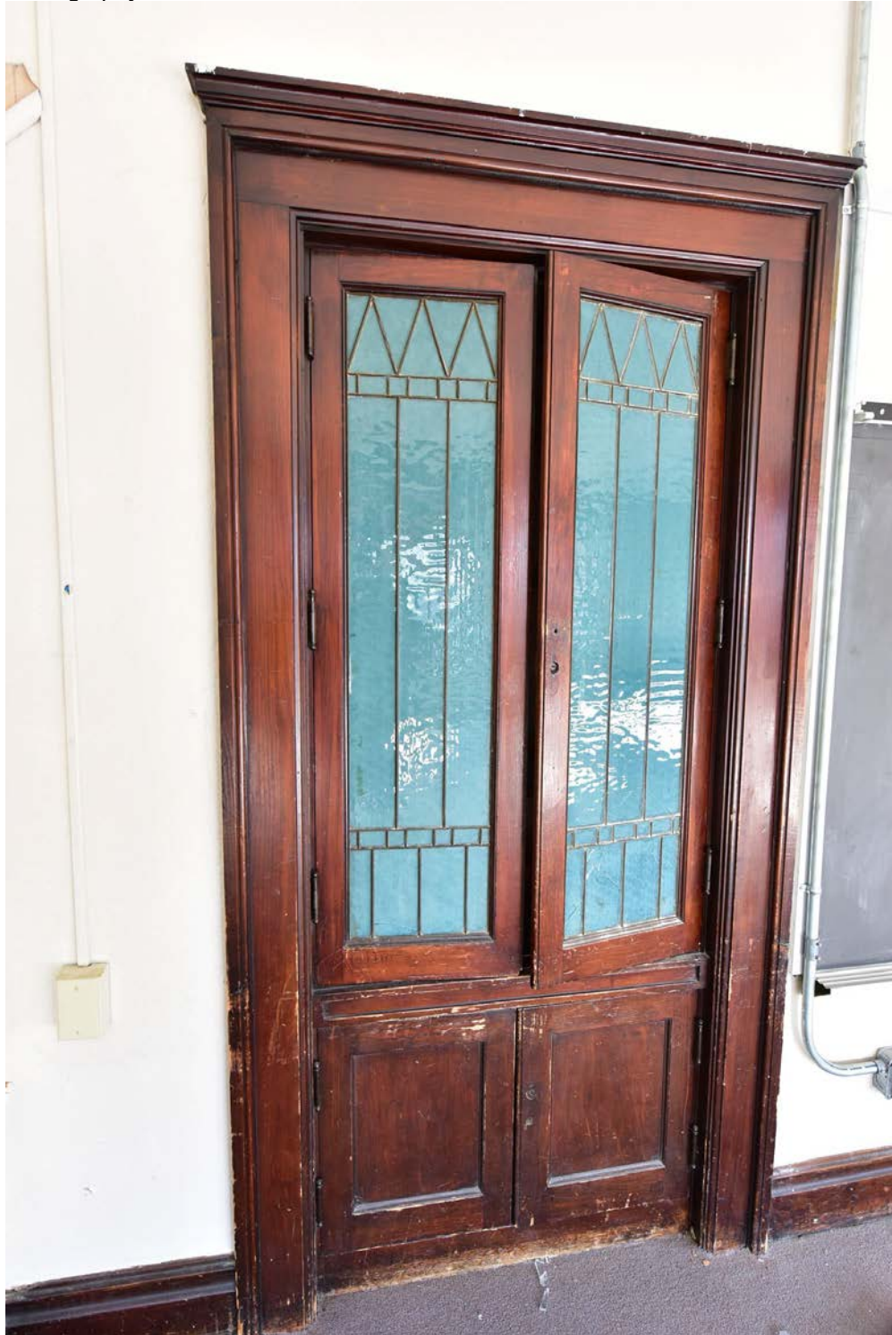
Figure 18. Photo of leaded glass doors for built-in cabinets in 1912 classrooms. Source: f-stop Photography, December 2020.
