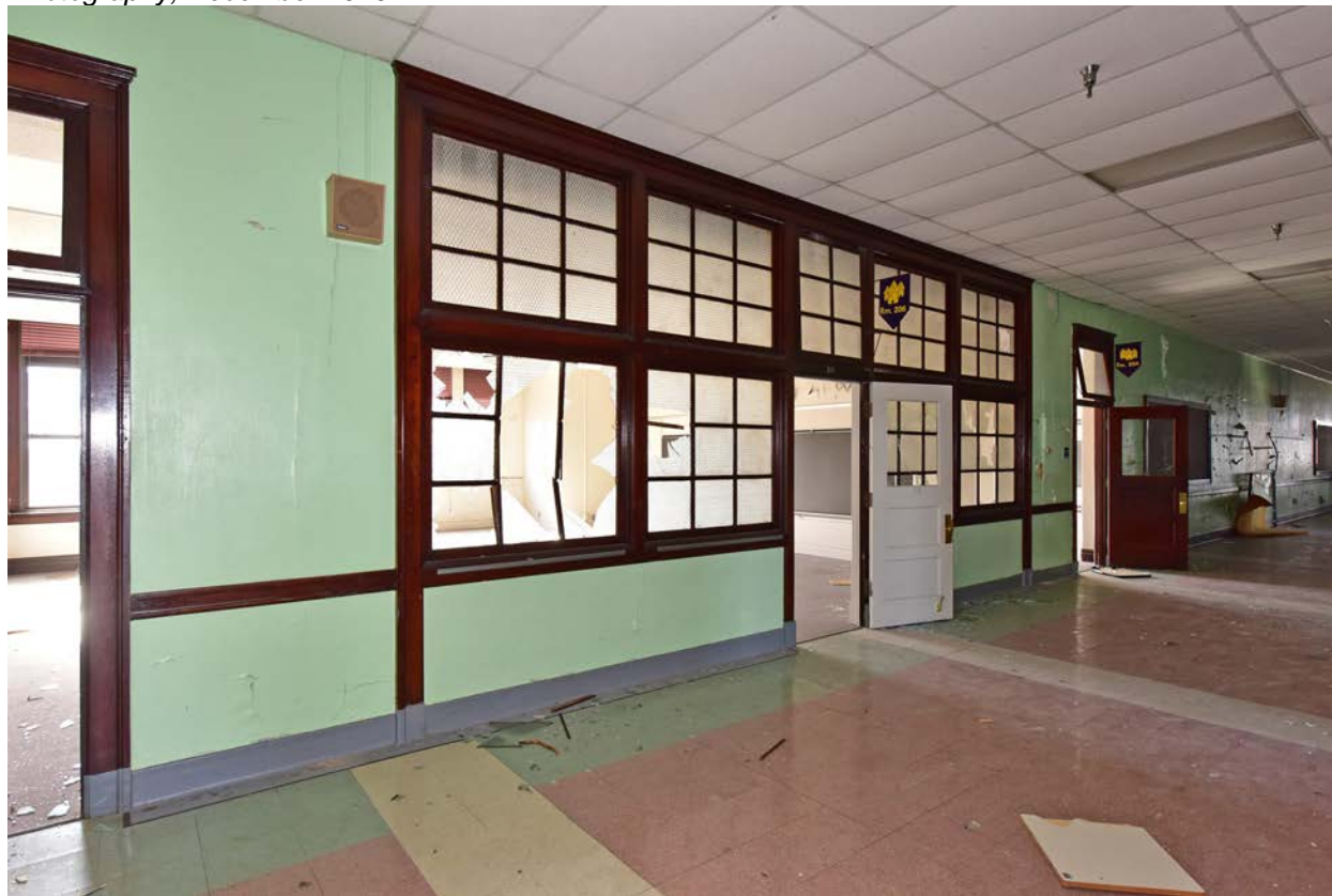
Figure 19. Photo of historic window wall on south side of second-floor corridor. Source: f-stop Photography, December 2020.
