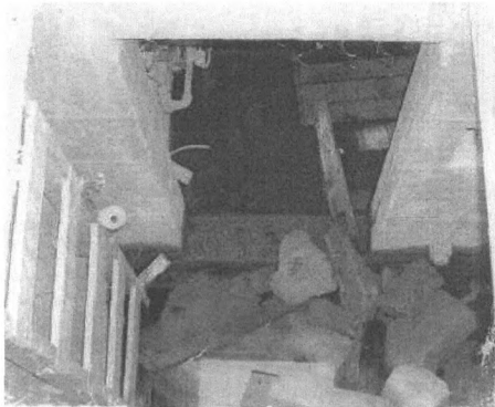
Equipment Vault (T-603), contributing structure, interior view from top of hatch, looking down.
