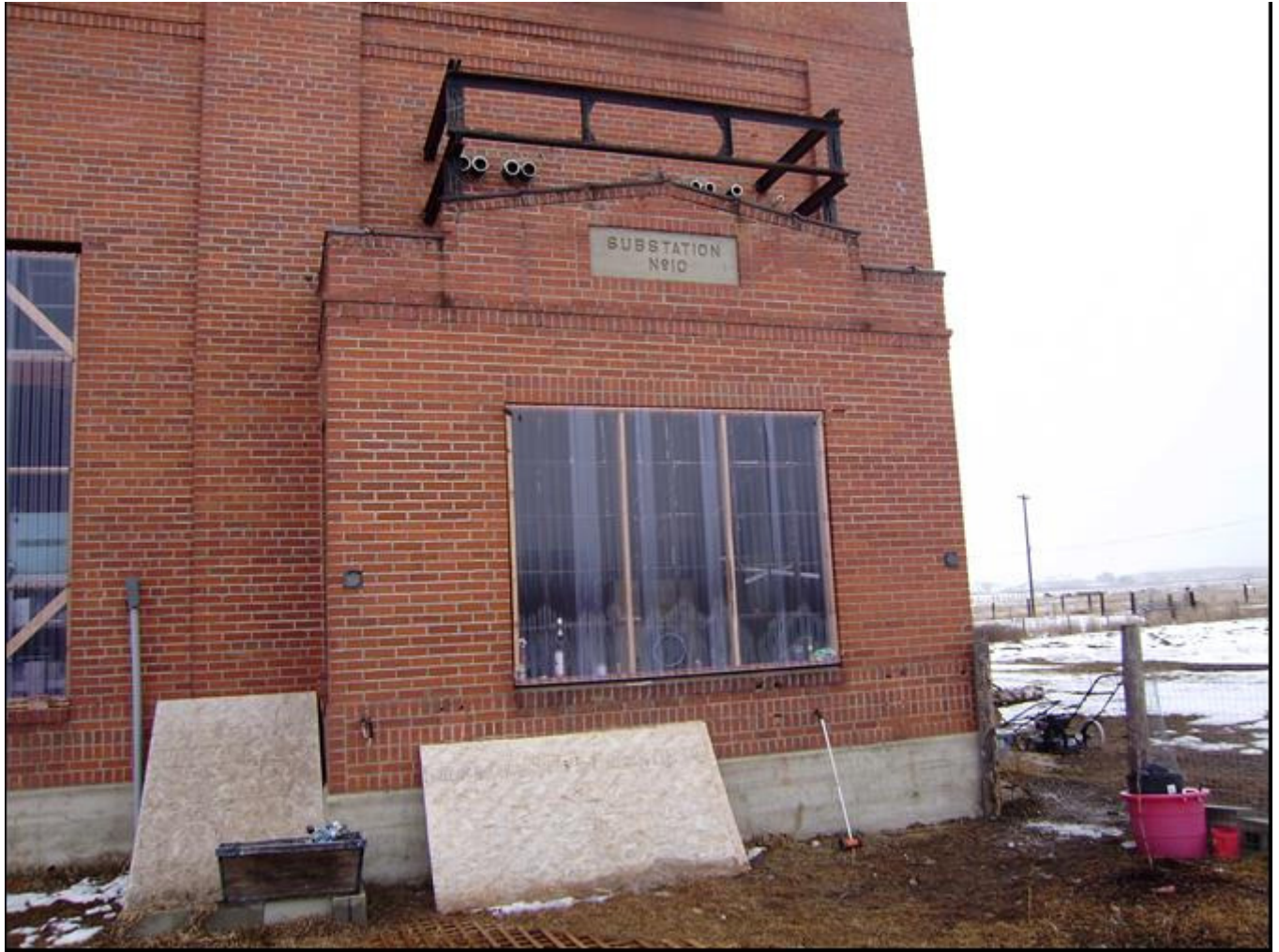
Photo 0008. Detail of substation operator's office. View to the north northeast.
