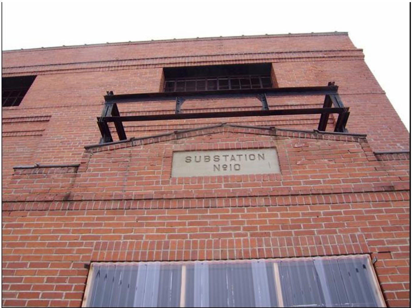
Photo 0009. Detail of substation designation and catenary support. View to northeast.
