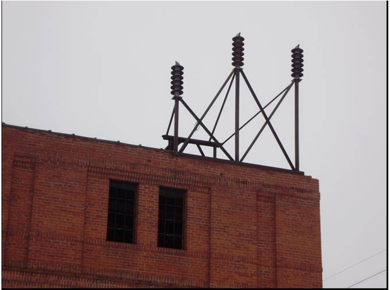
Photo 0017. Detail of lightning arrestors. View to southeast.
