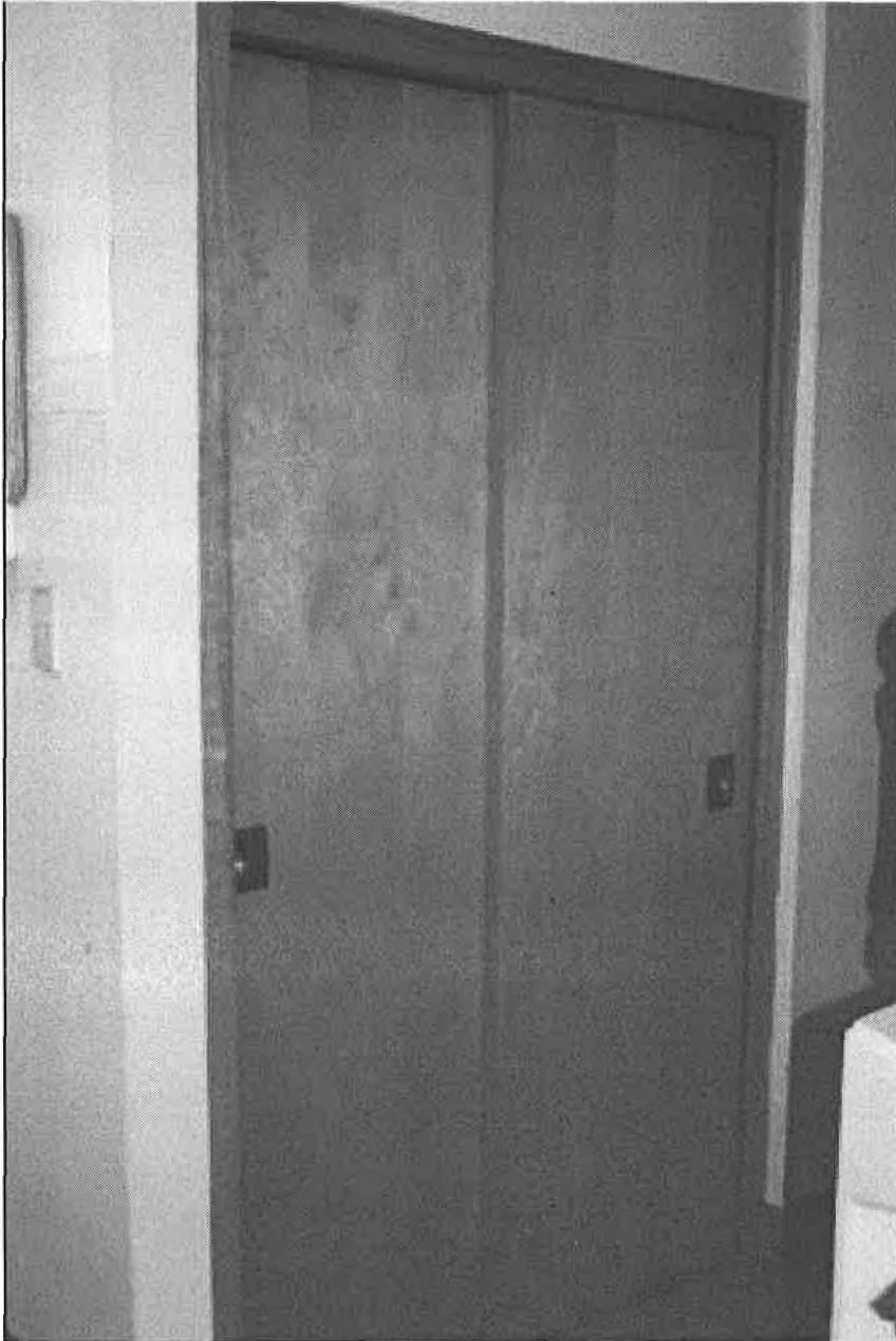
First floor coat closet with birch veneer sliding closet doors with inscribed brass pull plate.
