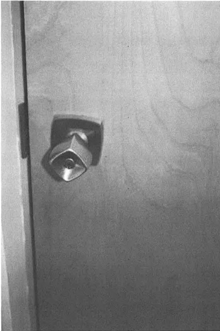
First floor, mechanical room, detail of birch veneer door and square brass knob.
