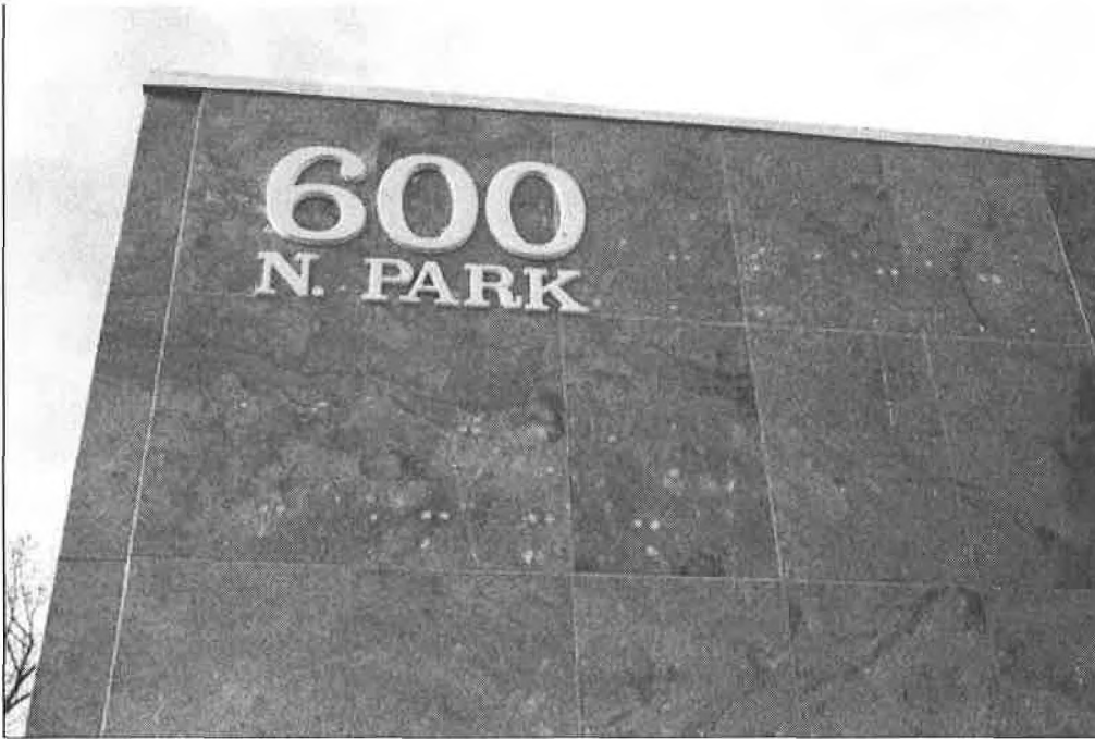
Photo 0010: East façade, pink granite detail, showing some damage where “Western Life” lettering was removed.
