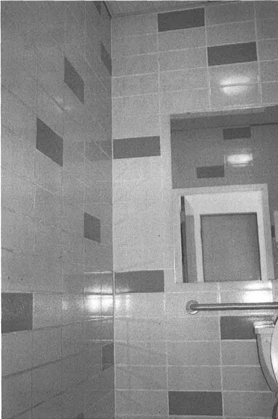
First floor, studio/guest room bathroom, view of peach and red structural glazed tile.
