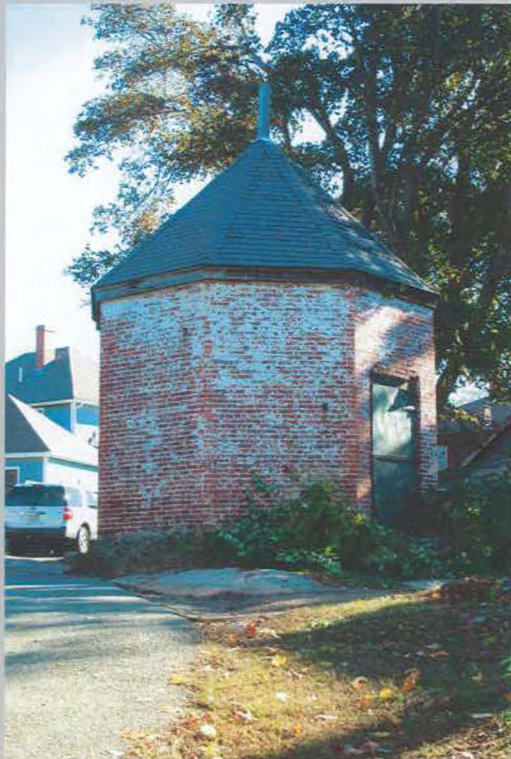
1. View E from Powder House Lane. Note ventilation holes in brick walls.
