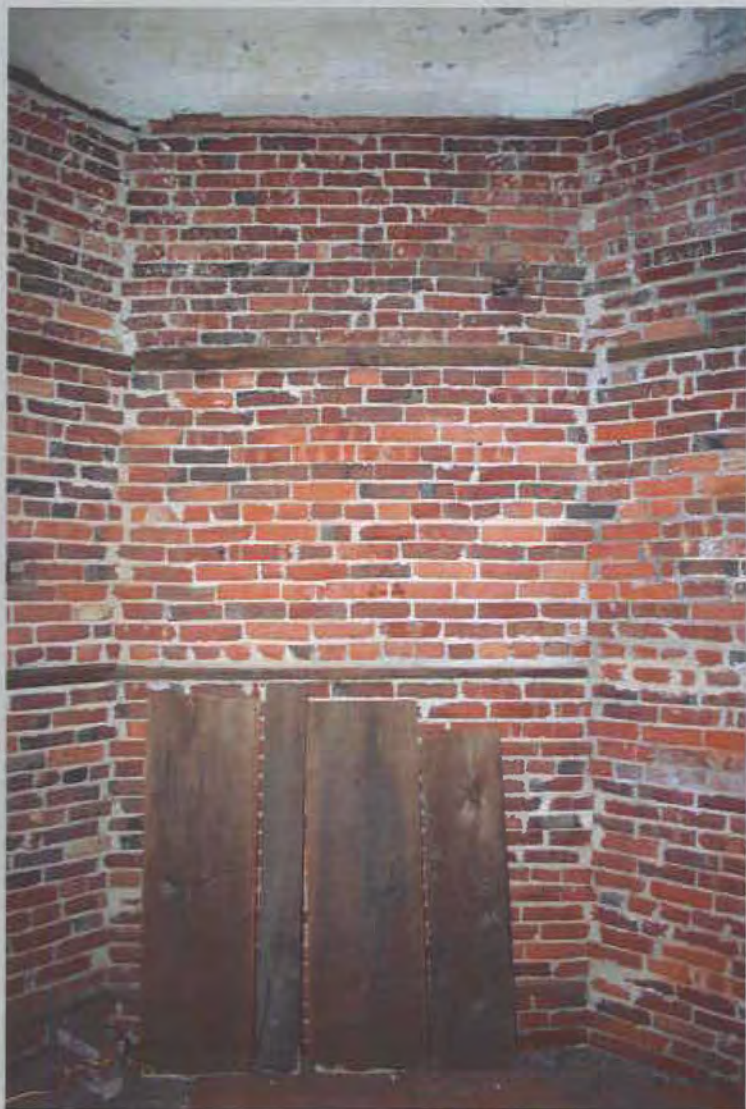
11. Interior detail showing remnants of nailers and wood liner (no longer attached). View NW.
