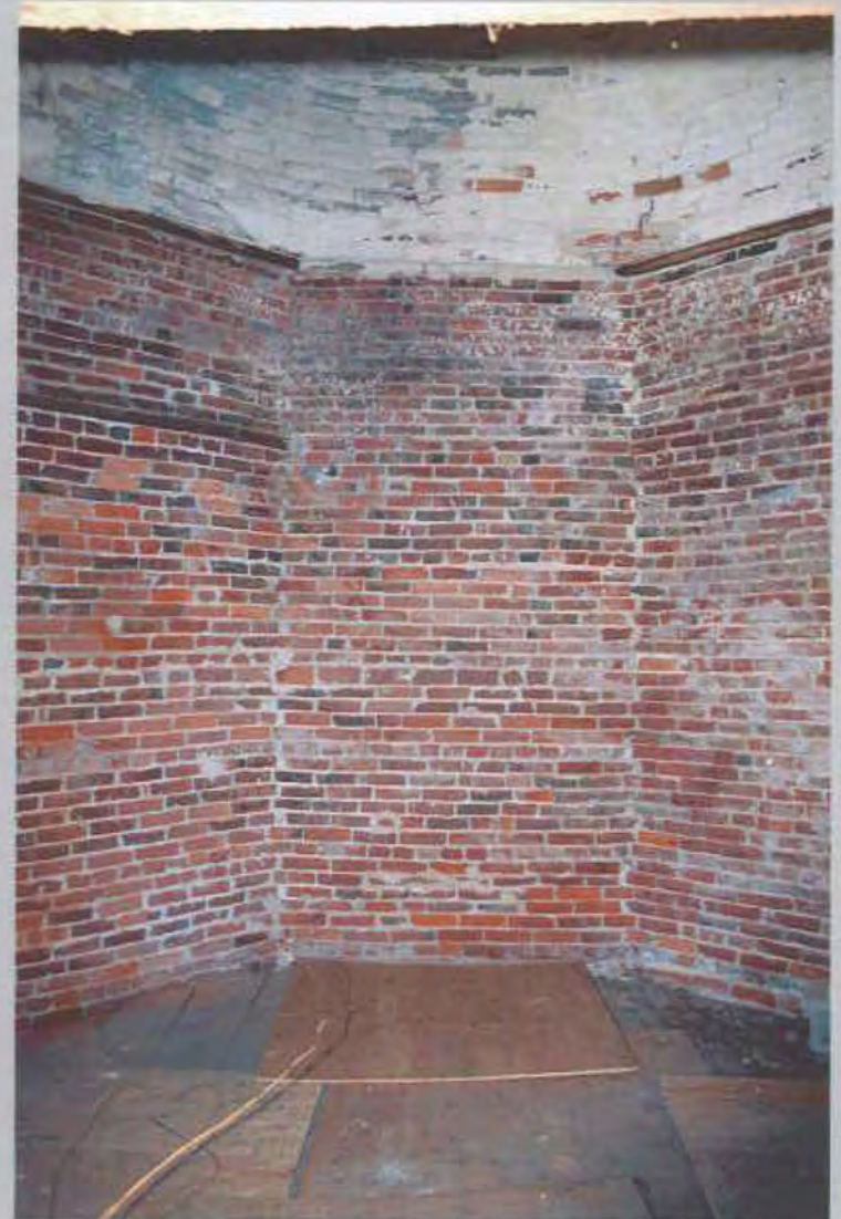
10. Interior detail showing juncture of dome with walls, and remnants of nailers for wood liner. View NE.
