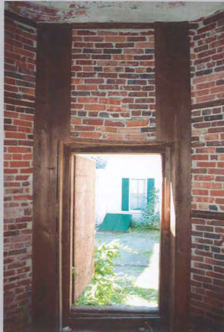
6. Interior detail of entry wall. View SW with adjacent house at 15 Madison Avenue in background.
