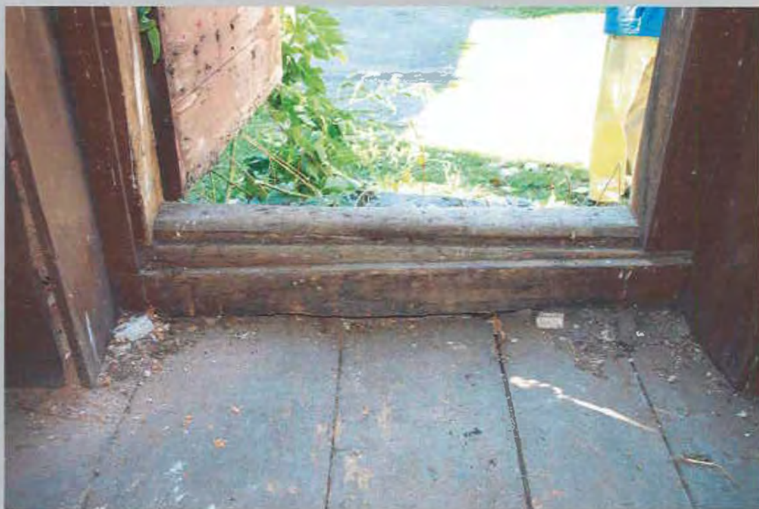
12. Interior detail showing floor, threshold, and bolts on interior of entry door. View SW.
