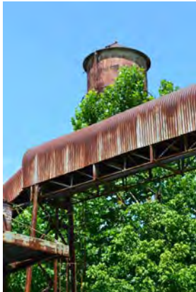
South and North Elevated Case Conveyors (41 & 42)
