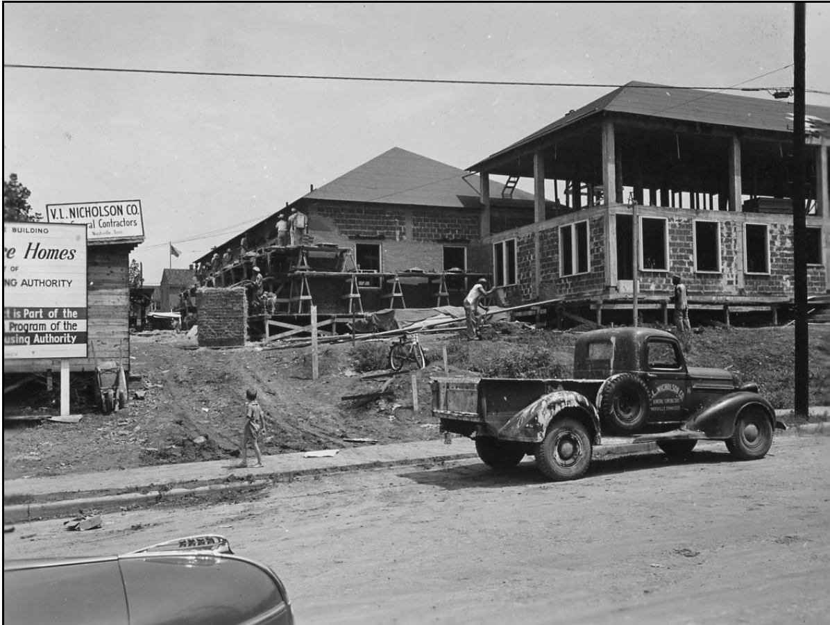
Figure 1. Construction of the James A. Cayce Administration Service Building in 1942. (Metro Nashville Archives)
