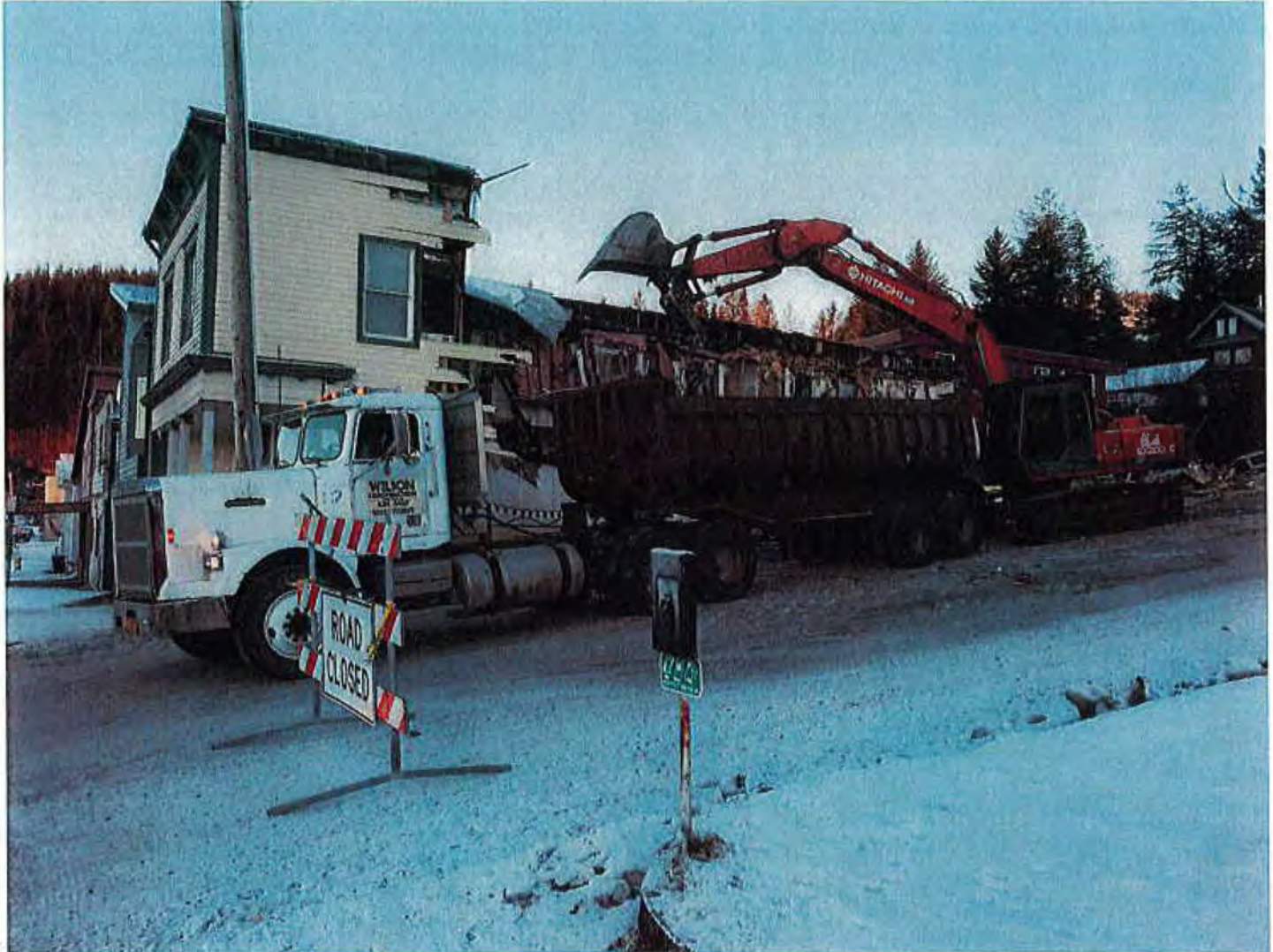
By late afternoon on Jan. 7, 2019, much of the demolished Reception Building had been hauled away in Wilson Construction dump trucks. (Photo by Dick Shellhorn/The Cordova Times)
