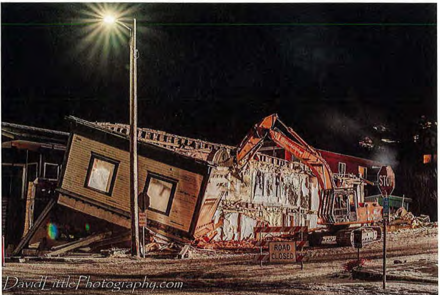
The historic Reception Building gets demolished. (Photo by David Little/for The Cordova Times)
