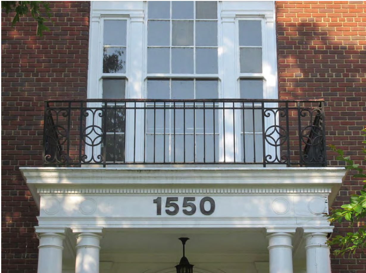
Detail of wrought iron balcony above entrance portico that incorporates the Chinese coin motif
