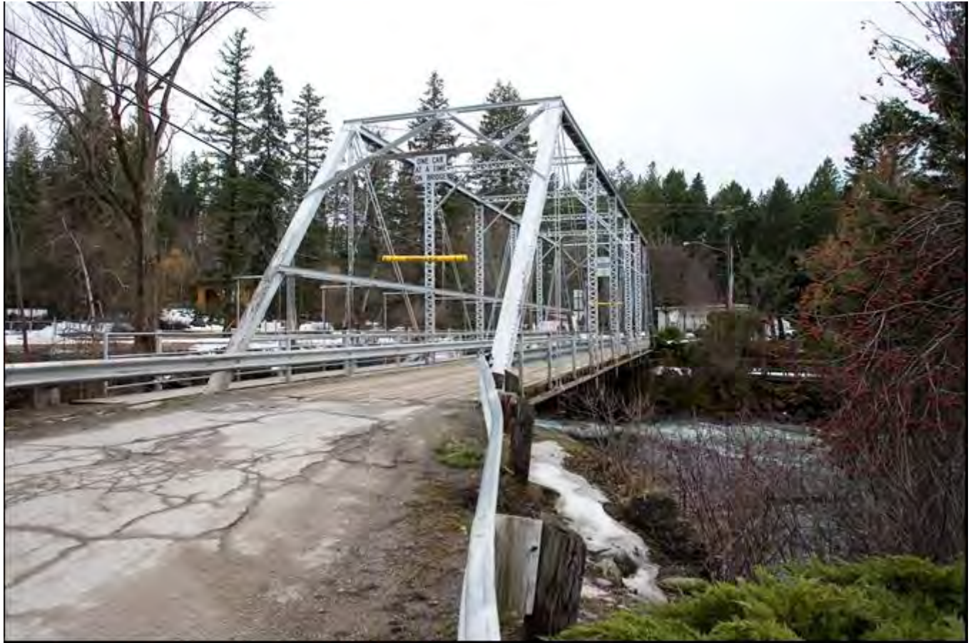
Photo 0003. Northeast portal and northwest side of the bridge. View to the southwest.
