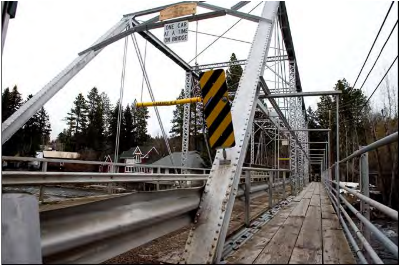
Photo 0006. Detail of sidewalk on southeast side of the bridge. View to the northeast.
