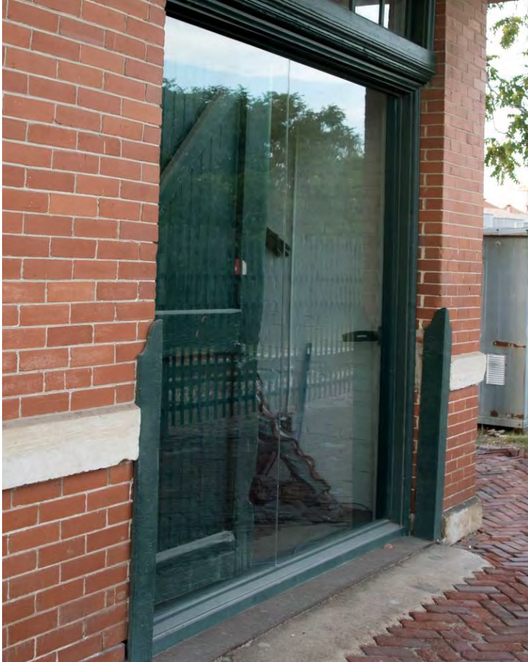
Photo 9: Baggage Room door detail—camera facing north northeast showing door inside fixed glass
