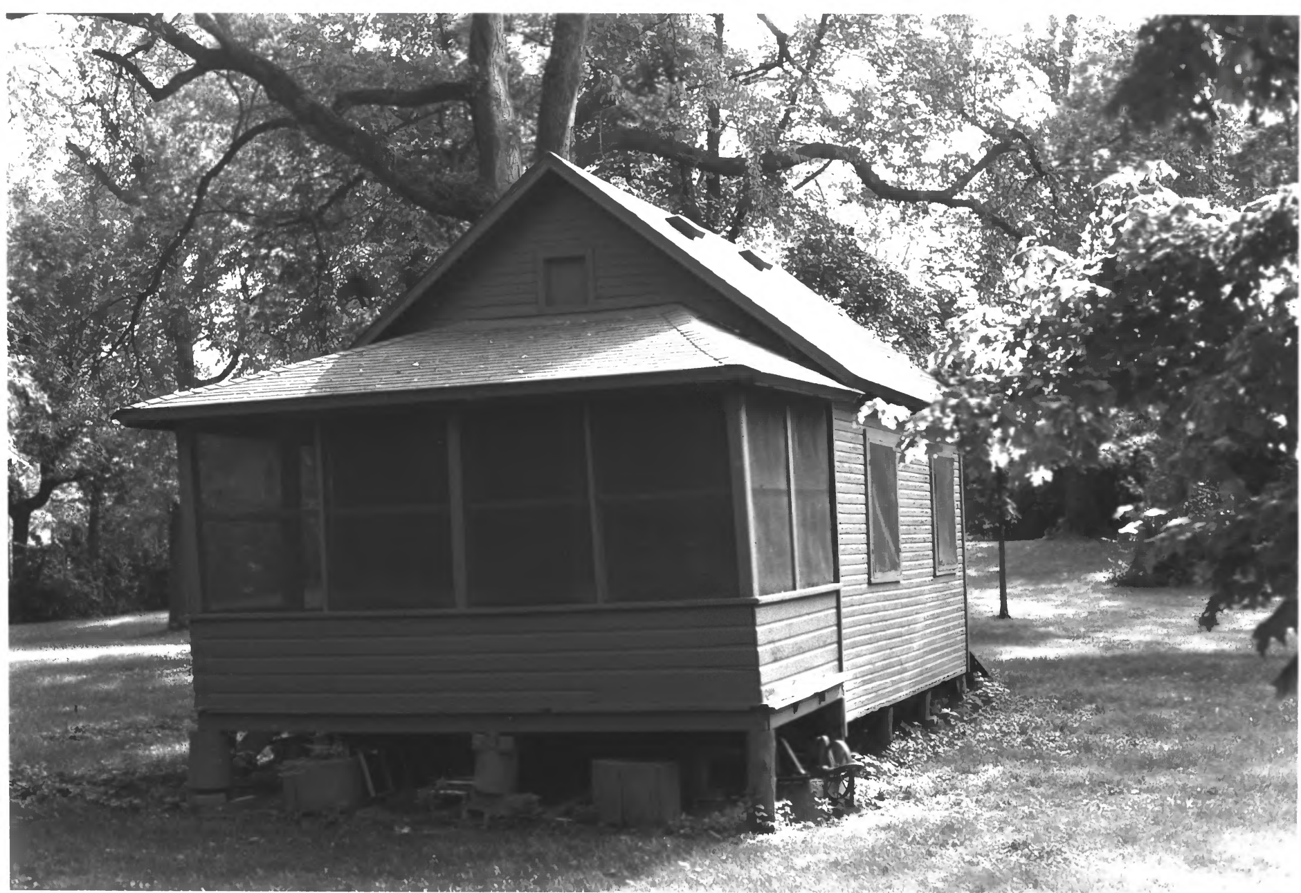
CARETAKER'S COTTAGE, CENTRAL COMMONS CRANE ISLAND HISTORIC DISTRICT HENNEPIN CO., MN. PHOTO I.D. # 010863-19
