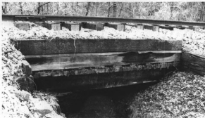
Figure 14: Located between mile marker 353 and 354 is a small steel girder and wood bridge typical of the smaller bridges built in the early 1900s to span small unnamed streams.
