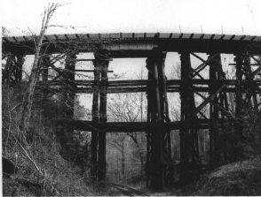
Figure 21: View of the railroad line and the trestle that loops above it.
