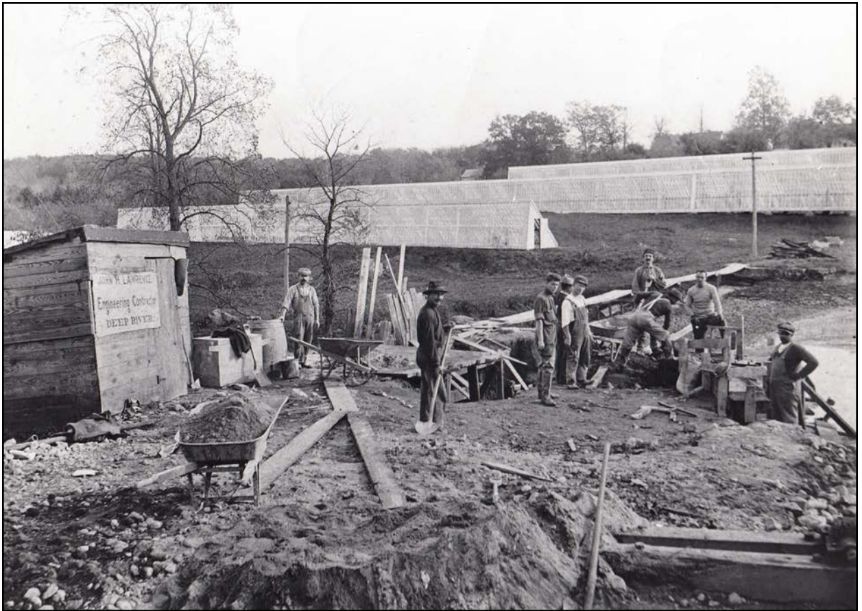
Figure 7. Building Dam at Lower Factory, ca. 1915—Note Bleach houses in background (Deep River Historical Society)
