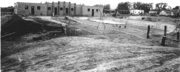
Looking NW at nearly complete bath house and swimming pool in progress, June 10, 1938
