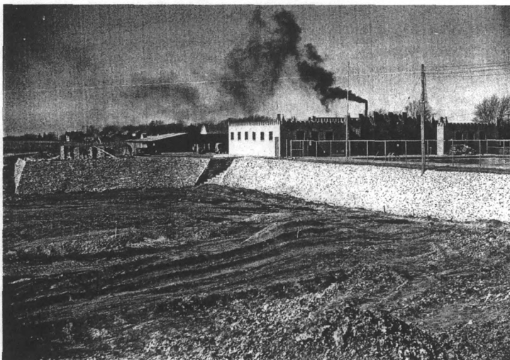
Looking NW at NW stone retaining wall, bath house and pool in background, and stone piers for pavilion in left-center February 24, 1939
