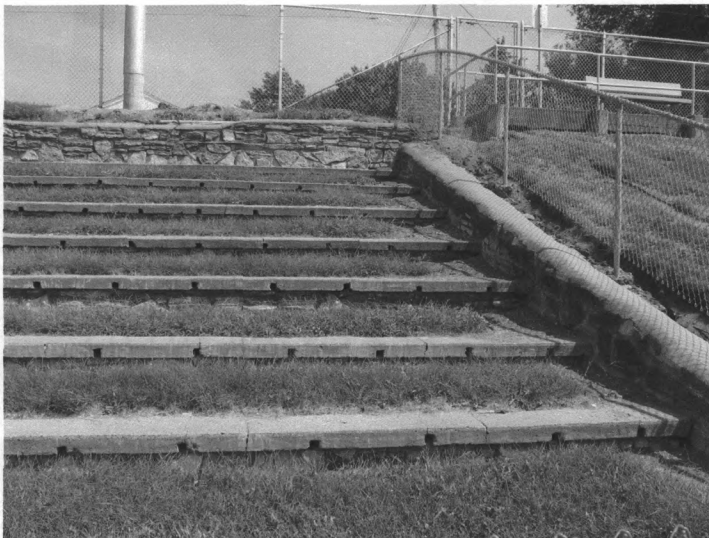
Detail of east-side bleachers showing drain holes under original concrete caps on the stone benches
