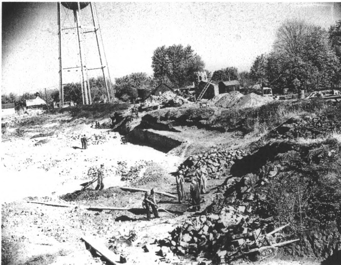
Looking NE at east side bleachers and gateway under construction with water tower in background October 14, 1938
