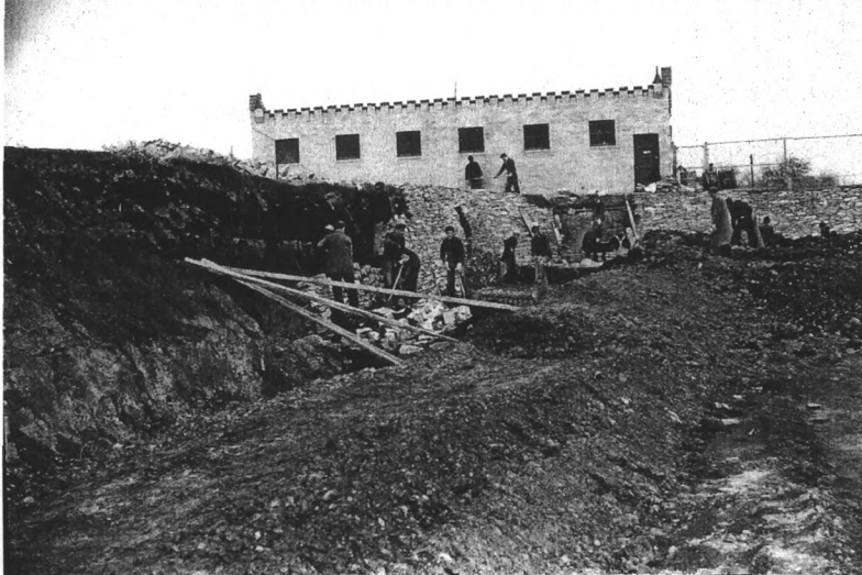
Looking North at NW stone wall under construction with pool house in background, November 17, 1938
