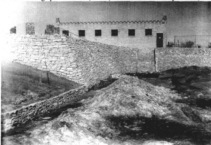
Looking North at NW stone retaining wall, bath house in background, and stone piers for pavilion in upper left February 24, 1939
