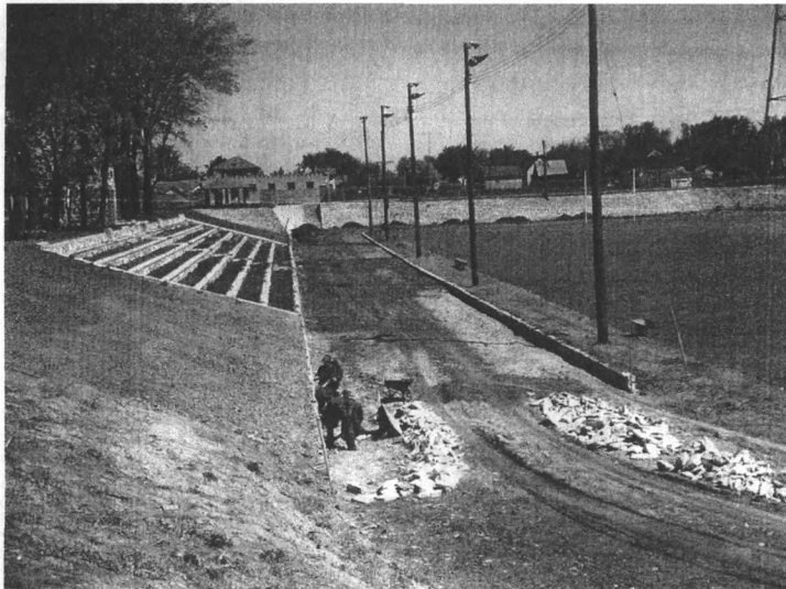
Looking North at cinder track construction along west side of field, May 16, 1940 (Note pavilion is now fully built in upper left-center of photo)
