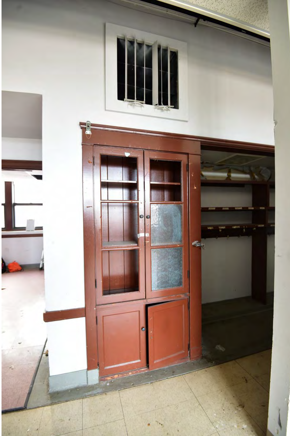
Figure 15. Historic ventilation system. Source: Brad Finch, 2017.
