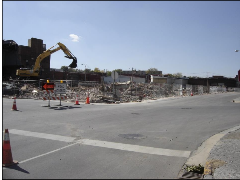
Figure 14: View to the east along the south side of West King Street which originally had the rear elevations of the frontages along West Market Street. Photo taken from the northeast corner of West King Street and North Boone Street. Photo dated 10/16/2012
