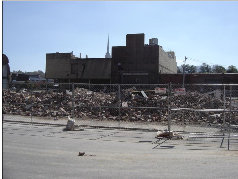
Figure 20: View to the south of the rubble of the resources. Photo dated 10/16/2012.
