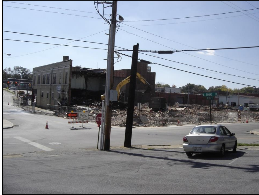
Figure 18: Demolition of 200 West Market Street. View is to the south of the rear (north) elevation. Photo dated 10/16/2012.
