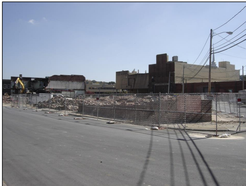
Figure 21: View to the southeast of the previous location of 104 Montgomery Street. Photo dated 10/16/2012.
