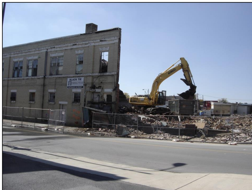
Figure 19: Demolition of 200 West Market Street. View is to the northwest of the south façade. Photo dated 10/16/2012.
