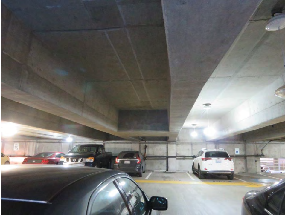
Photo 28 of 28. WA_King County_Freeway Park 0028. Ceiling of Freeway Park Garage, above which is located Freeway Park's East Plaza, view east.
