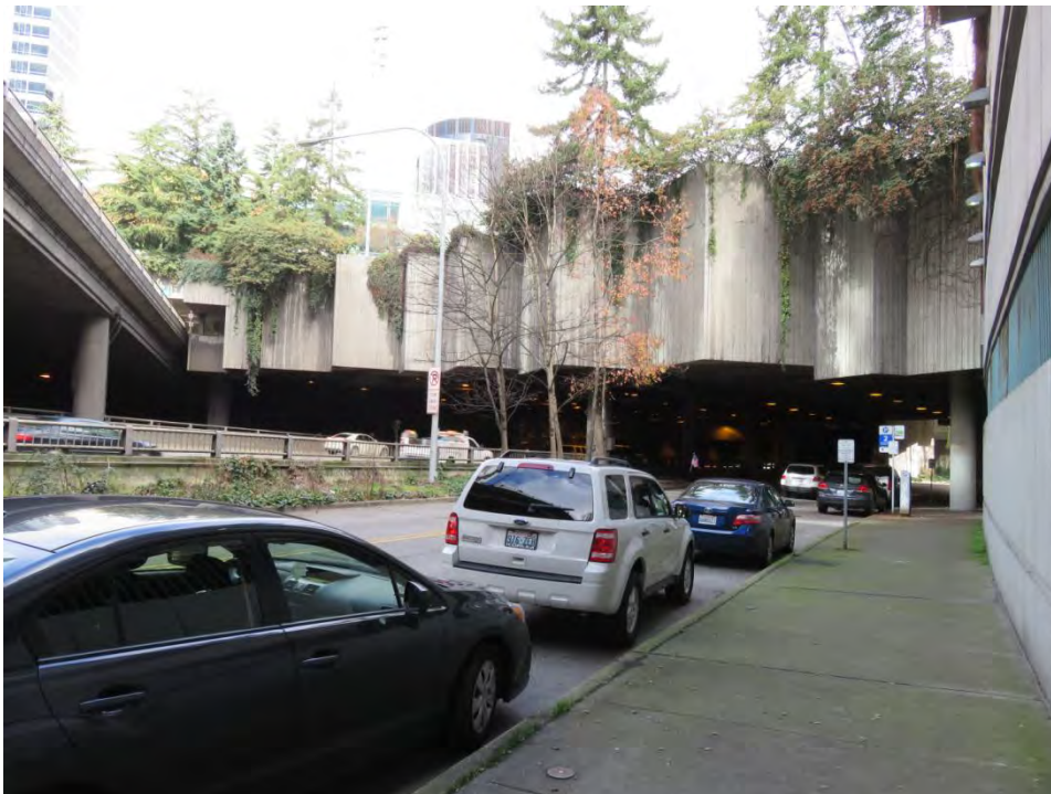
Photo 25 of 28: WA_King County_Freeway Park 0013. The planters of Freeway Park and WSCC, viewed from Hubbell Pl., view northeast.
