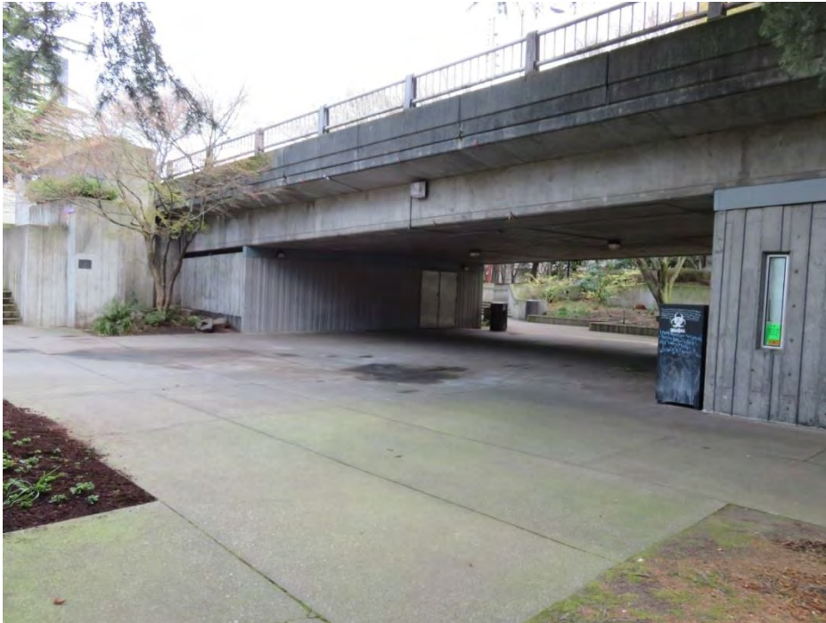
Photo 14 of 28: WA_King County_Freeway Park 0015. 8 th Ave. as it passes above Freeway Park and noncontributing maintenance sheds, view to the north.
