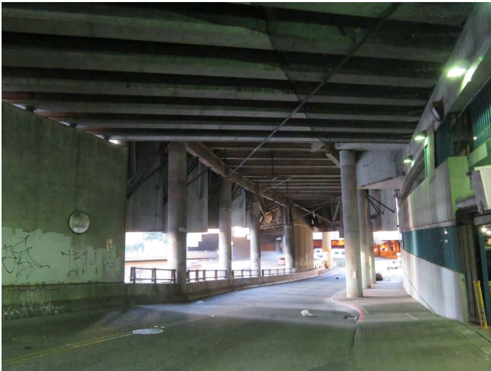
Photo 23 of 28. WA_King County_Freeway Park 0024. Approach to Freeway Park Garage from Hubbell Pl., entrance to the right, view north.
