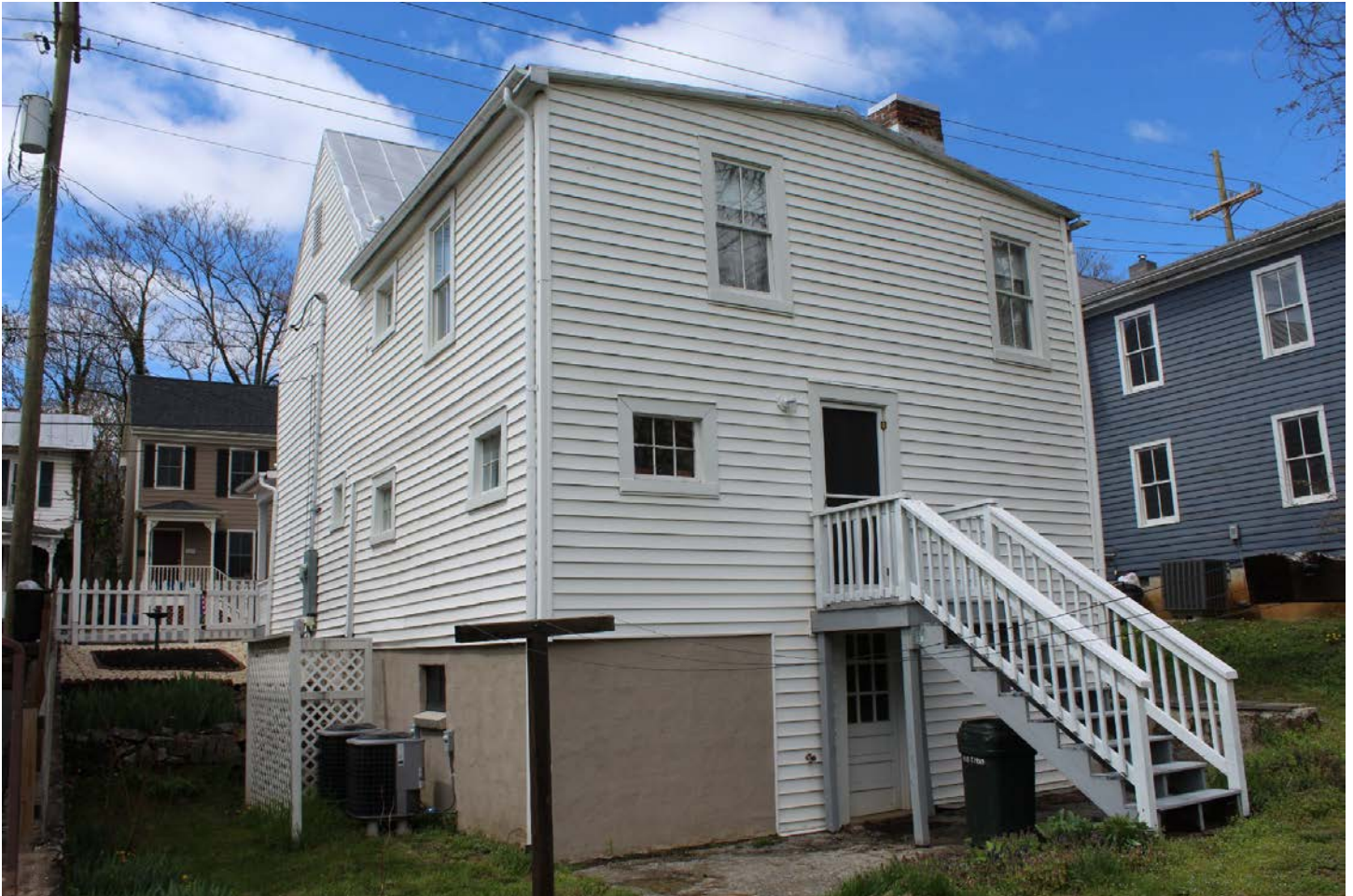
Photo 4. Exterior, looking northwest from backyard, showing side garden and south and east elevations. April 2018.
