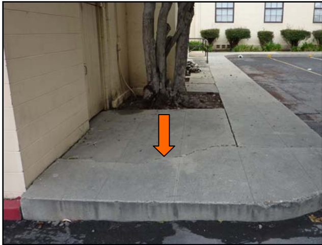
Cracks and buckling in concrete paving are a tripping hazard, and direct water to building foundations.
