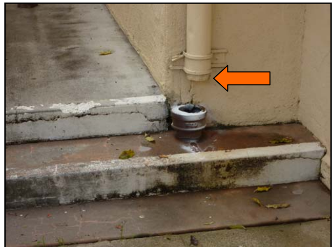
Downspouts no longer connect to many of the drainage leaders.
