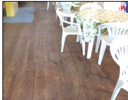
Oak flooring at the Balcony has minor water stains.
