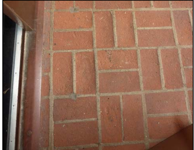
Hard and impermeable mortar is causing brick paving at the Vestibule to erode.
