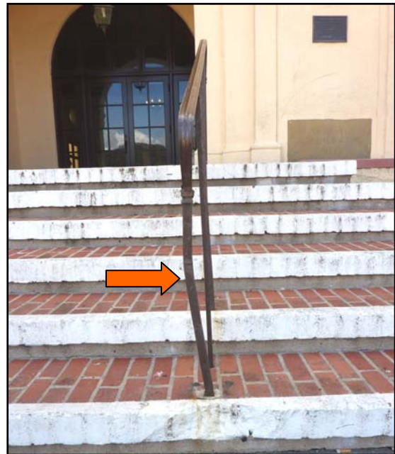
The west railing at the main entrance steps is deformed.
