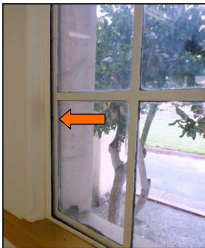
A steel casement window in the Banquet Hall does not fully close on the hinge side.
