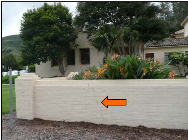
A large crack at the brick site wall indicates active deterioration.
