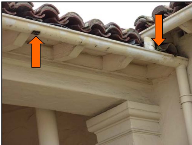
Isolated sections of gutters are rusted through, and weeds are growing in accumulated debris.
