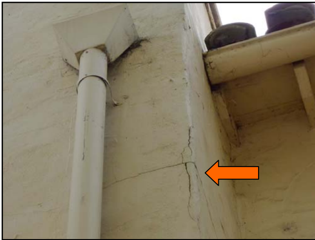
Wide cracks in the stucco at the Auditorium should be repaired to prevent moisture penetration to wood sheathing and framing.
