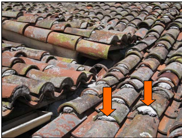
Mortar applied to roofing tiles during a previous repair are visually obtrusive (photo courtesy of Robert Ooley).
