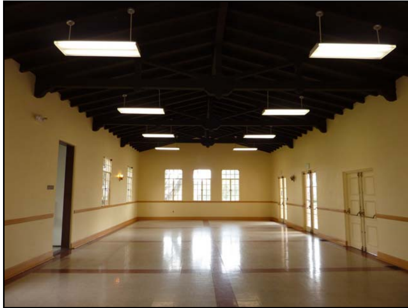
Suspended light fixtures in the Banquet Hall are replacements.
