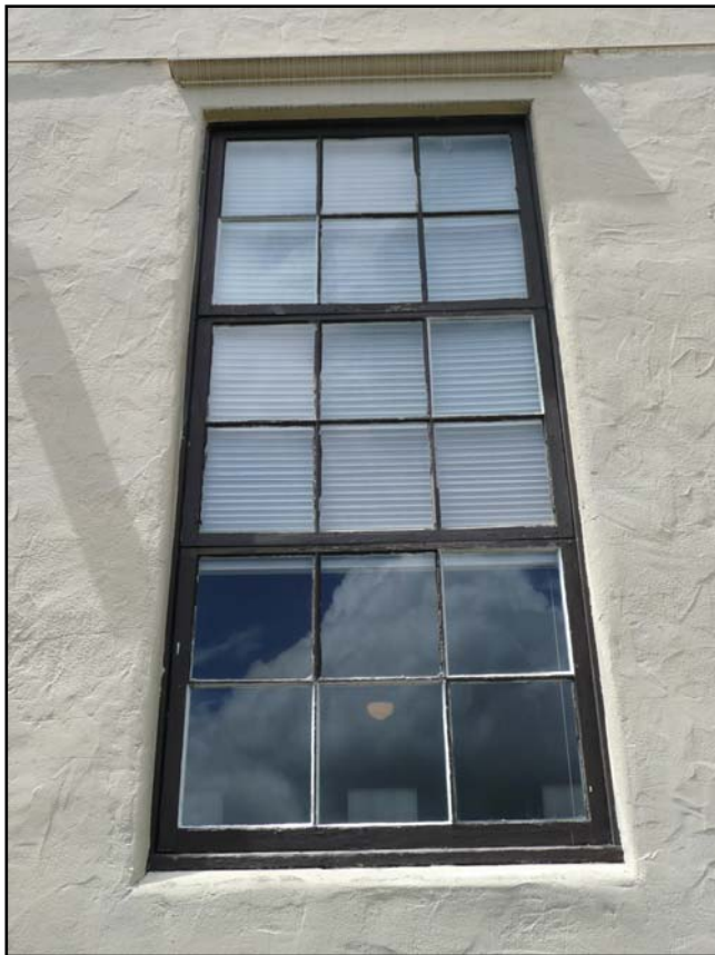
Triple-hung wood sashes at the Auditorium are warped and paint and glazing putty have failed.
