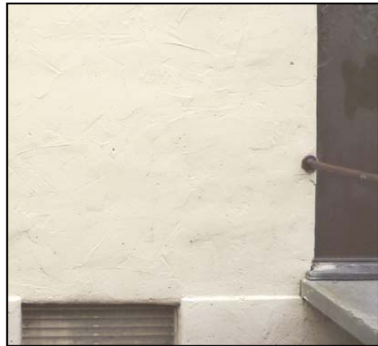
Small pocks and voids are evident throughout the stucco at the rear of the Stage.
