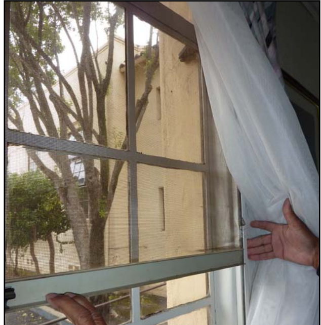
Retractable window screens are still present and operable in at least one historic office space in Room 138.
