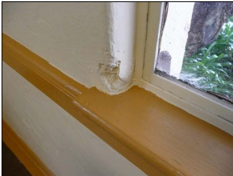
Casement windows in the Banquet Hall show damage to plaster at the lower corners.
