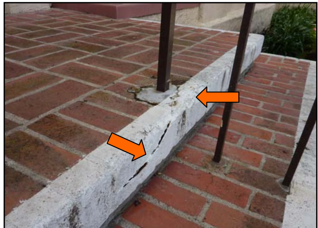
Corrosion of the iron railing at the main entrance is causing the brick steps to crack and spall.
