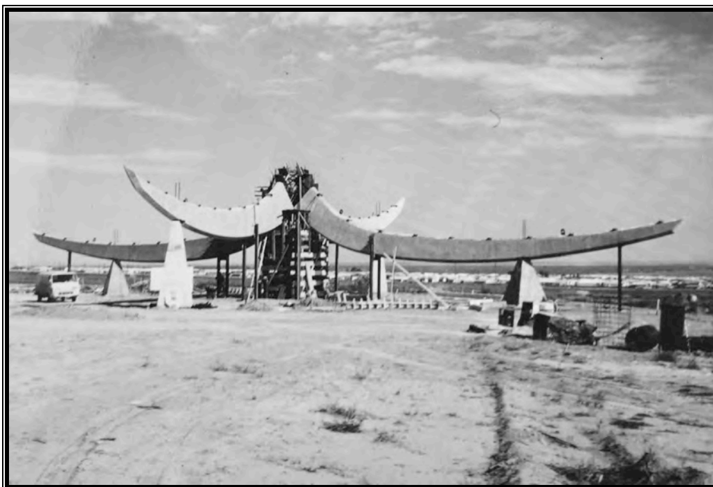
HP-2: All Four Roof Beams and Supports in Place, November 1963 (Courtesy of Joel Haertling)
