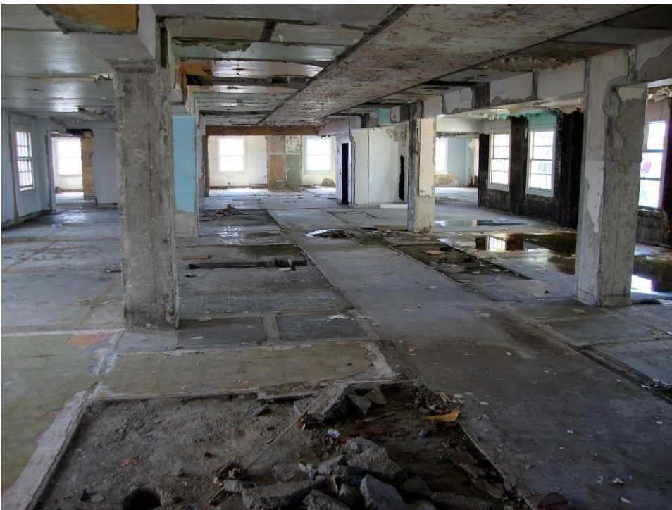
23 Typical floor plate showing evidence of room divisions; camera on third floor facing west.
