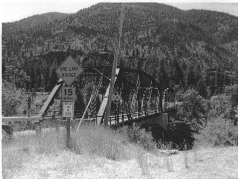
Photograph 002: West profile of truss spans and north portal. View to the southeast.
