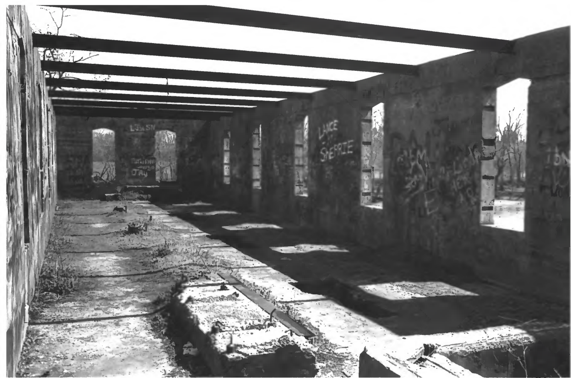
Harms Mill Hydroelectric Station Fayetteville vicinity, Lincoln Co., TN
