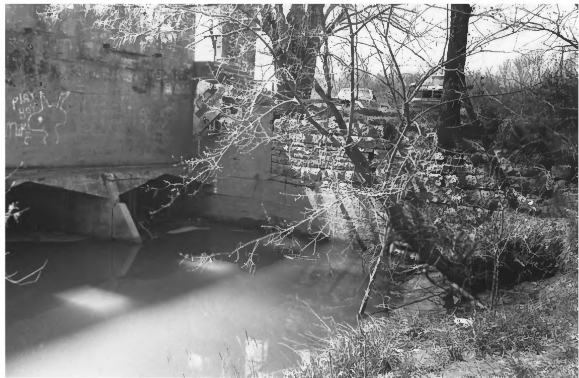
Harms Mill Hydroelectric Station Fayetteville, vicinity, Lincoln Co., TN
